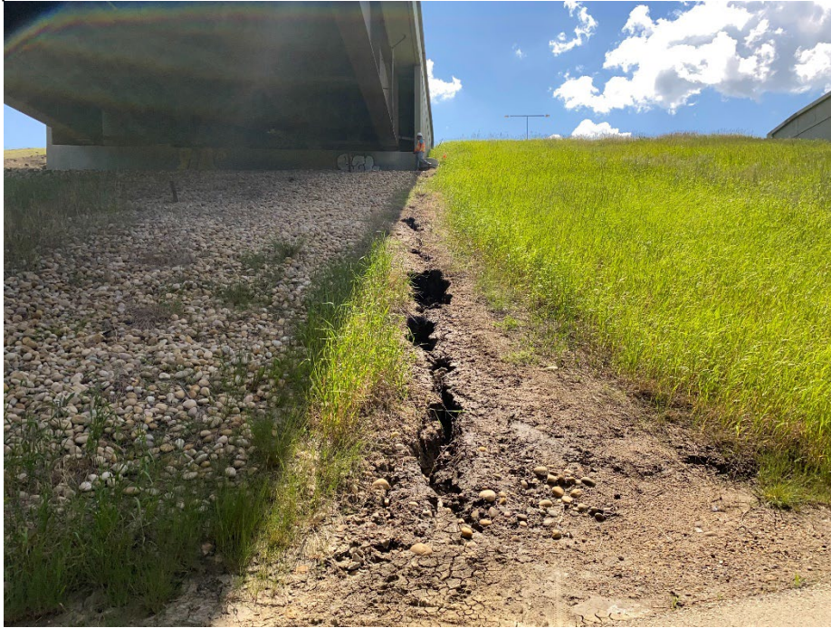
Photo 9: Erosion below the NB abutment on the south slope due to damaged waterproof membrane on abutment. Looking southeast.
