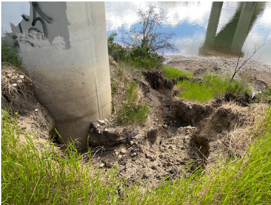
Photo 2: Loss of soil support at pier. Looking northeast.
