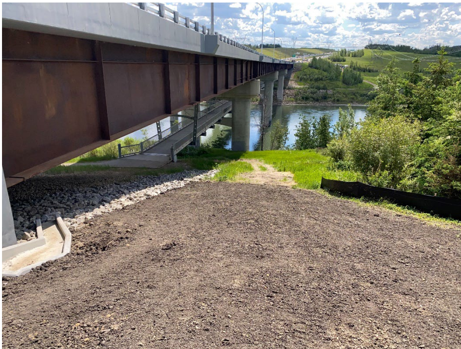
Photo 4: View from top of north slope, down to northwestern pier. Drainage trough installed at SBL north abutment. Looking southeast.
