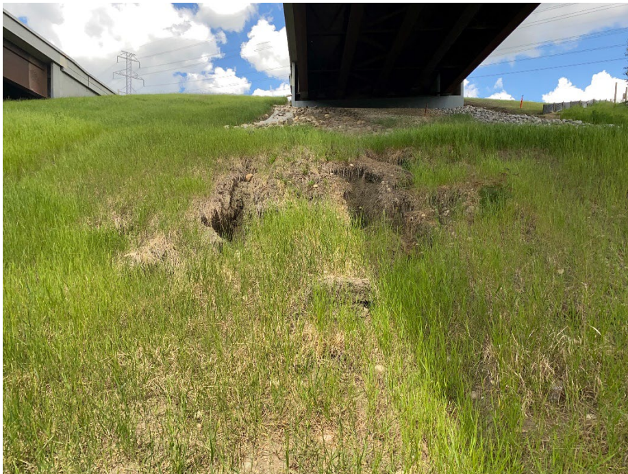
Photo 6: Four scour holes downslope of pedestrian trail under NBL. Looking northwest.
