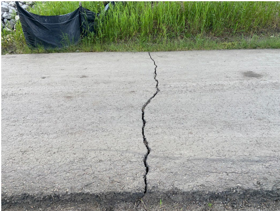
Photo 10: Crack in the paved trail below the NB lane of south abutment. Looking southeast.
