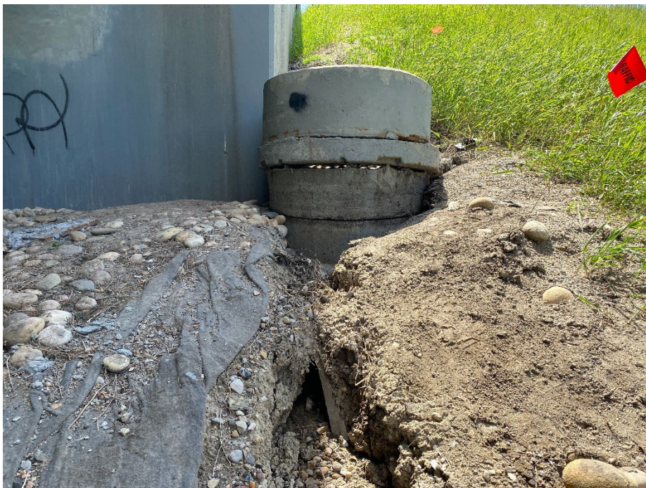
Photo 8: Catch basin on west side of NBL south abutment, not connected to an underground drainage system. Looking southeast.
