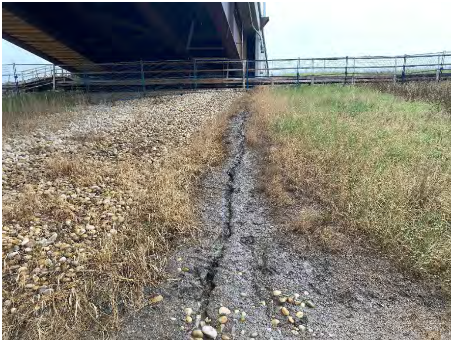
Photo 6: Erosion below the NB abutment on the south slope due to damaged waterproof membrane on abutment. Looking southeast.
