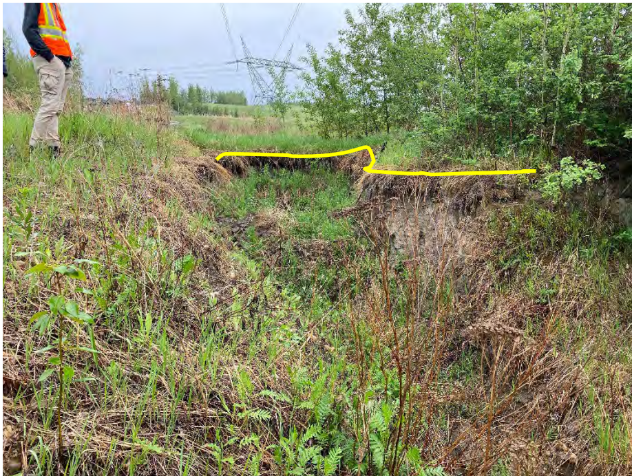
Photo 8: Two slumps adjacent and behind the outfall on the south bank of the river. Looking southeast.
