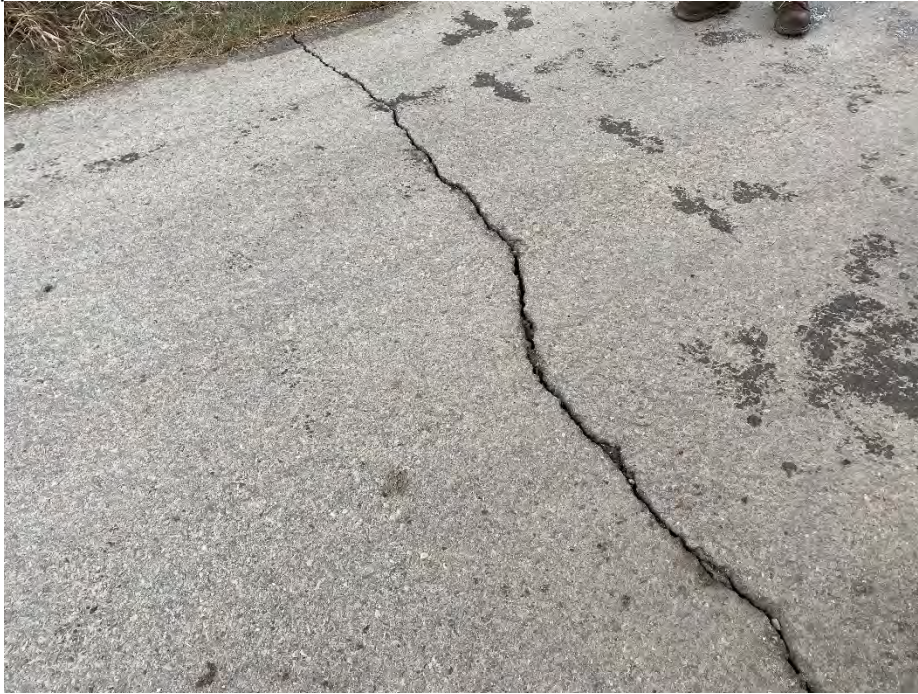
Photo 7: Crack in the paved trail below the NB lane of south abutment. Looking northeast.
