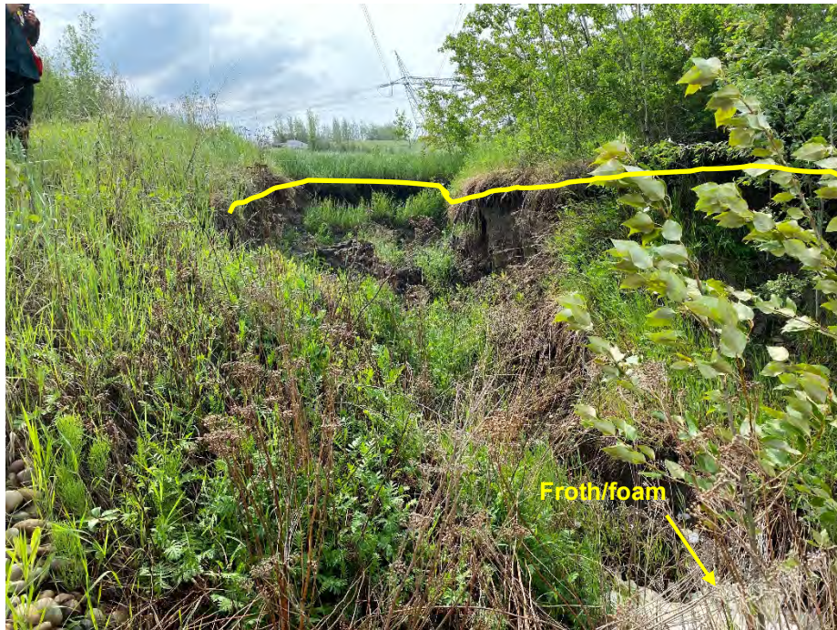
Photo 6: Two bowl shaped slumps adjacent and behind the outfall on the south bank of the river. Looking southeast.
