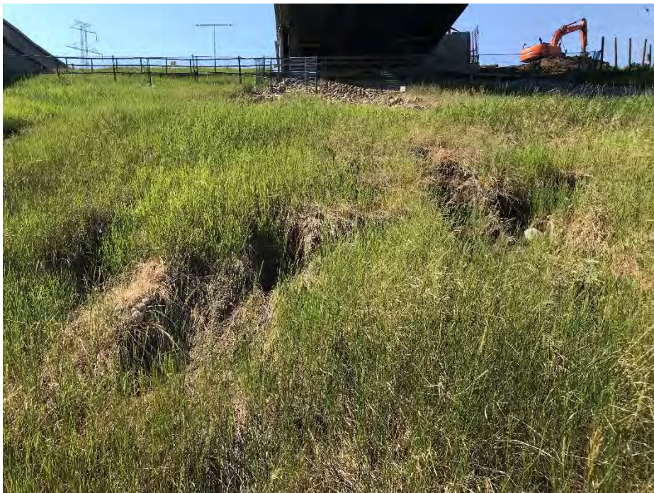
Photo 4: Four scour holes downslope of pedestrian trail under NBL. Looking northwest.
