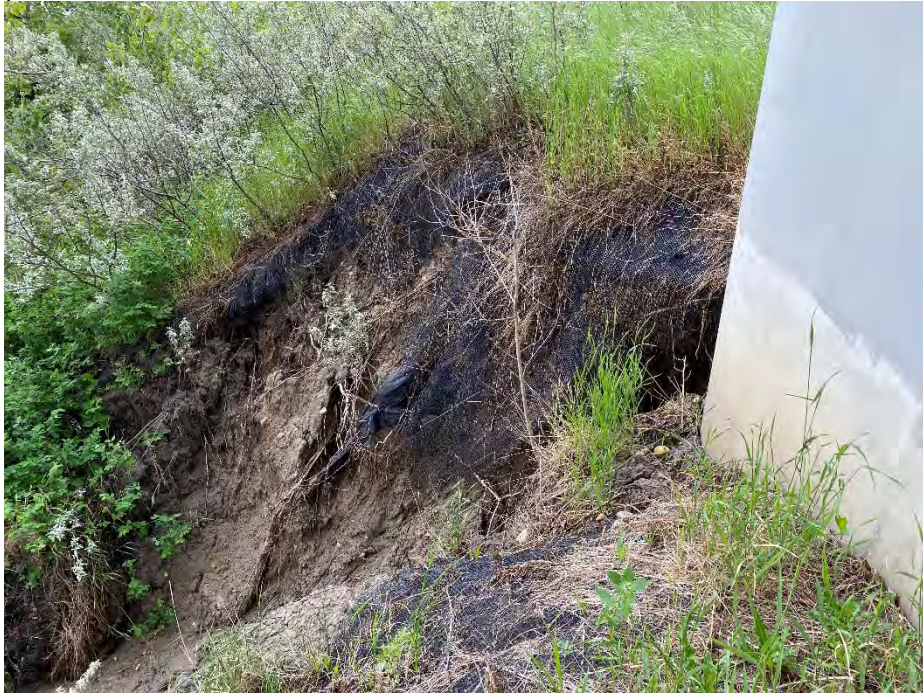
Photo 3: Erosion at outermost pier of southbound lane. Looking southwest.
