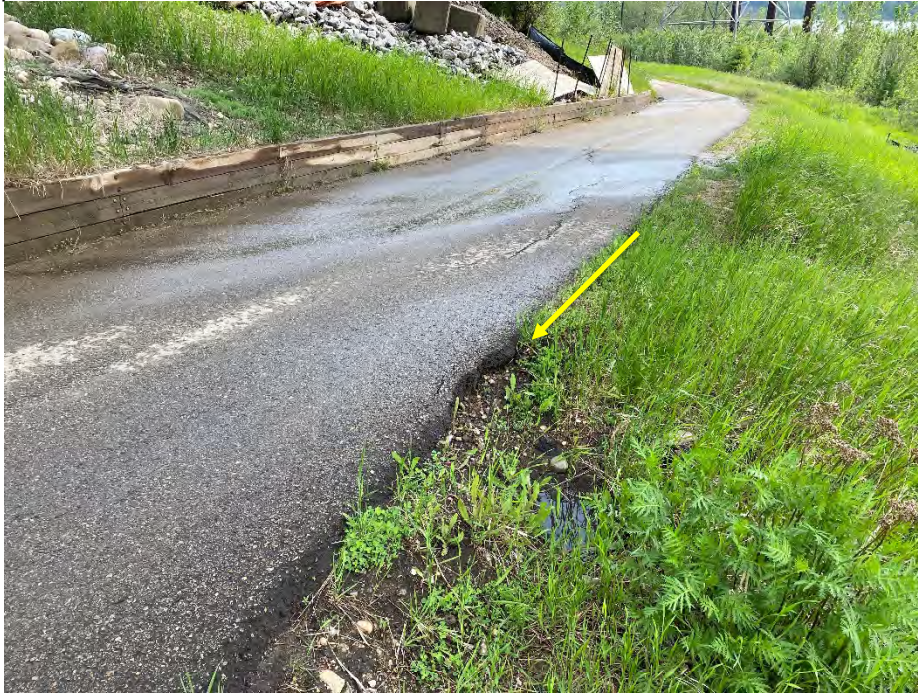
Photo 5: No change to trail crack pattern. Minor loss of trail. Looking northeast.
