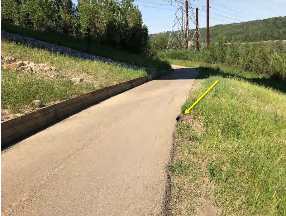
Photo 5: No change to trail crack pattern. Minor loss of trail. Looking northeast.
