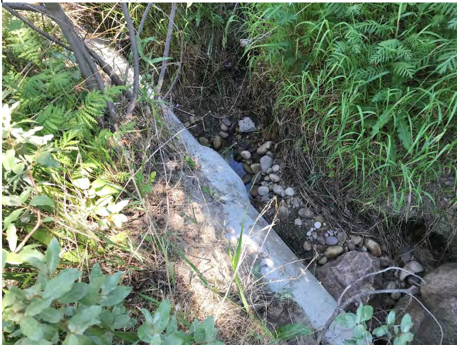
Photo 7: Water ponding below the separated pipe at the outfall. Looking down.
