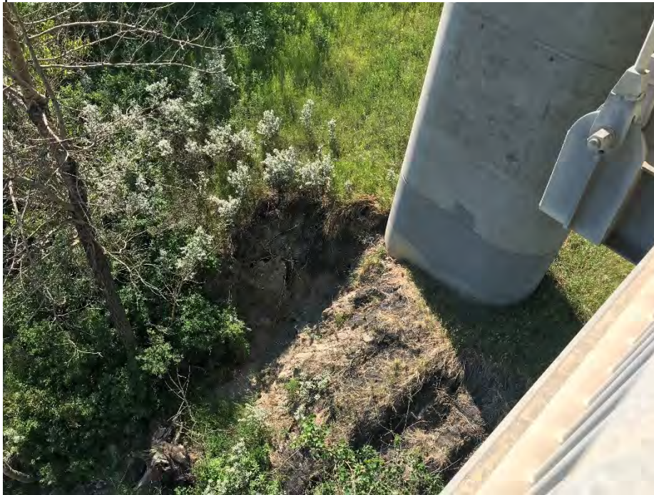
Photo 3: Erosion at outermost pier of southbound lane. Looking northwest.
