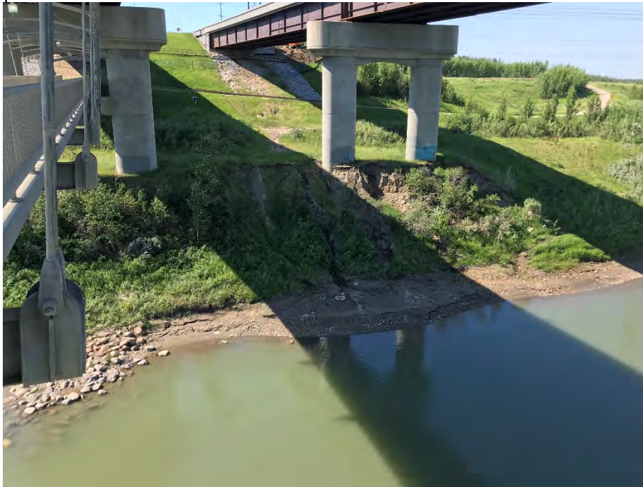
Photo 1: Erosion of land piers at the north bank. Looking north.
