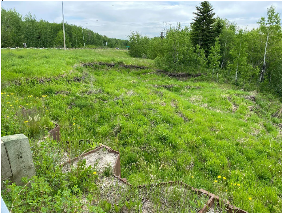
Photo 1: Slope movement downslope of pile wall. Looking northeast.
