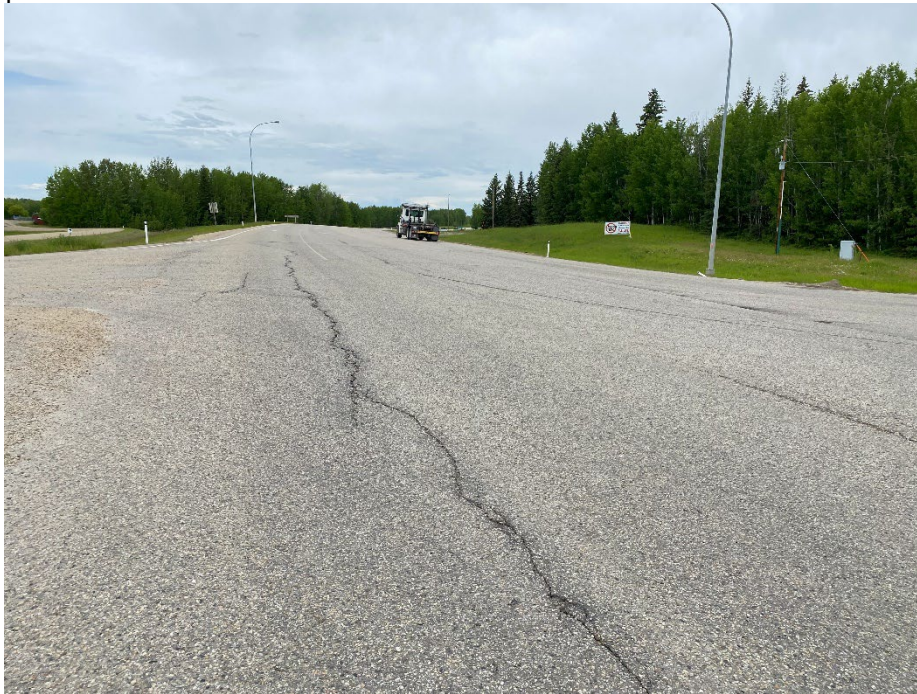
Photo 5: Pavement condition at intersection. Looking west.
