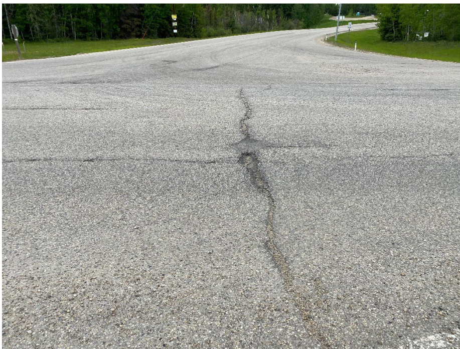
Photo 4: Crack on east side of intersection. Looking north.
