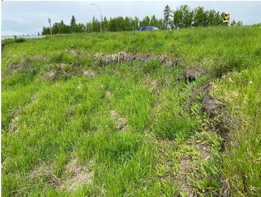
Photo 3: Vegetated scarp. Looking northeast.
