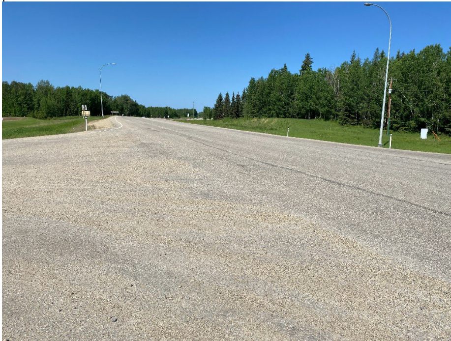
Photo 5: Pavement condition at intersection. Looking southwest.
