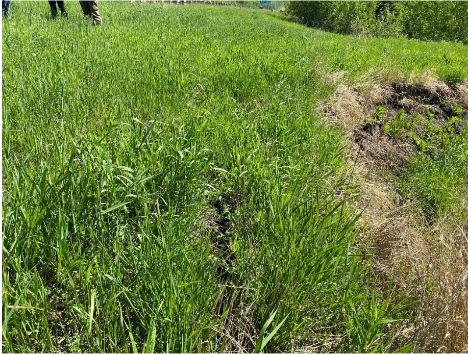
Photo 3: Tension crack upslope of the current scarp. Looking northeast.
