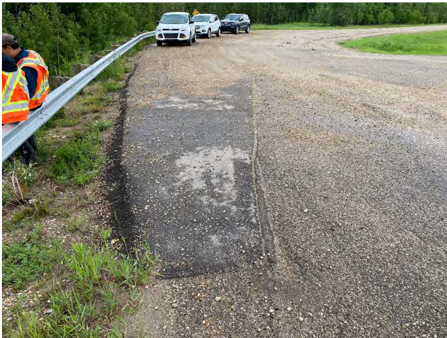
Photo 4: Separation of new and old pavement west of pile wall. Looking south.
