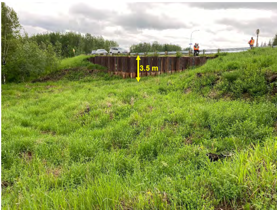
Photo 2: Slope movement downslope of pile wall. Looking southwest.
