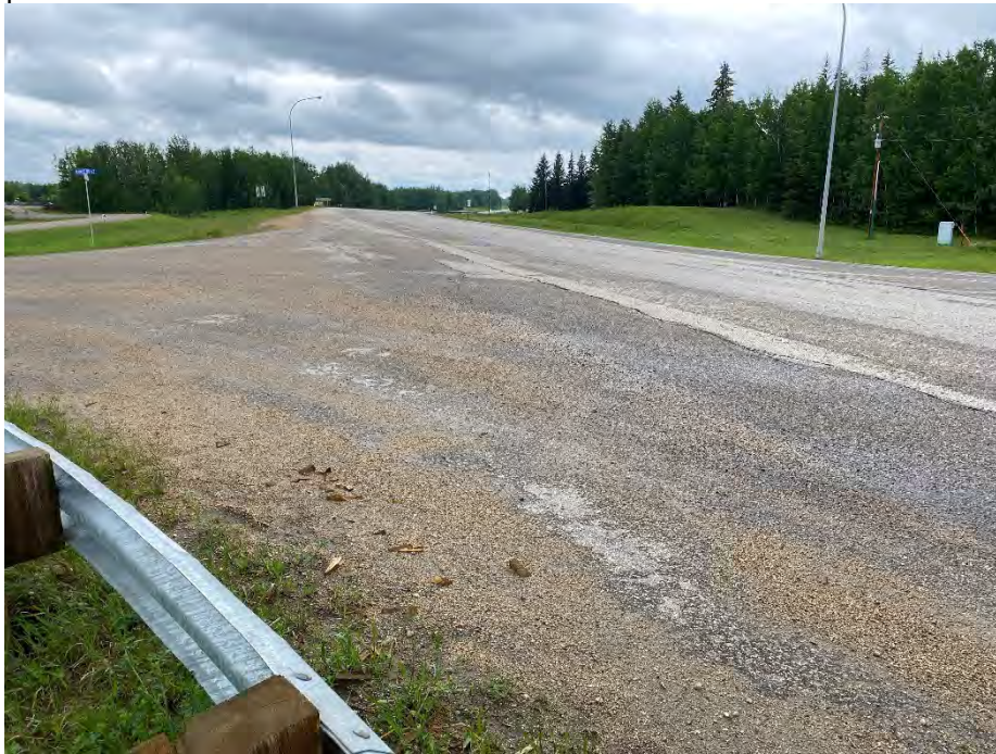
Photo 5: Pavement condition at intersection. Looking southwest.
