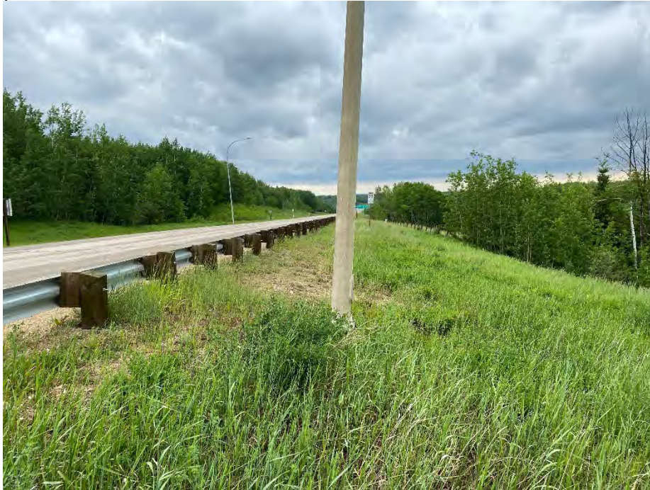
Photo 3: Leaning light standard. Looking northeast.
