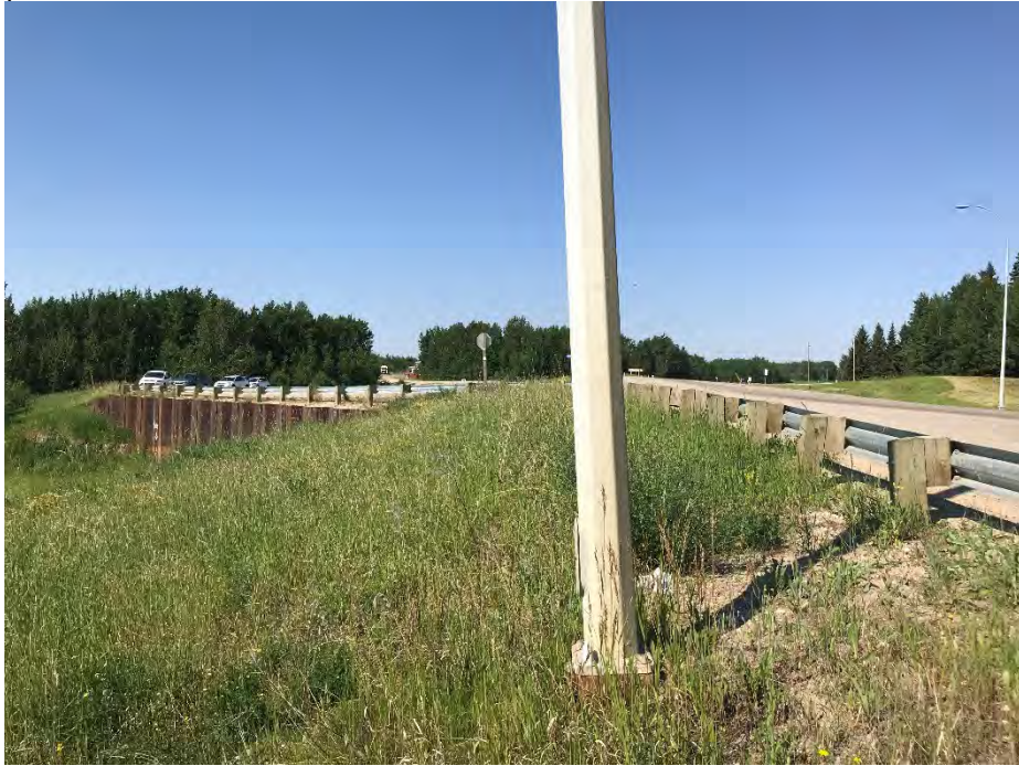
Photo 3: Leaning light standard. Looking southwest.
