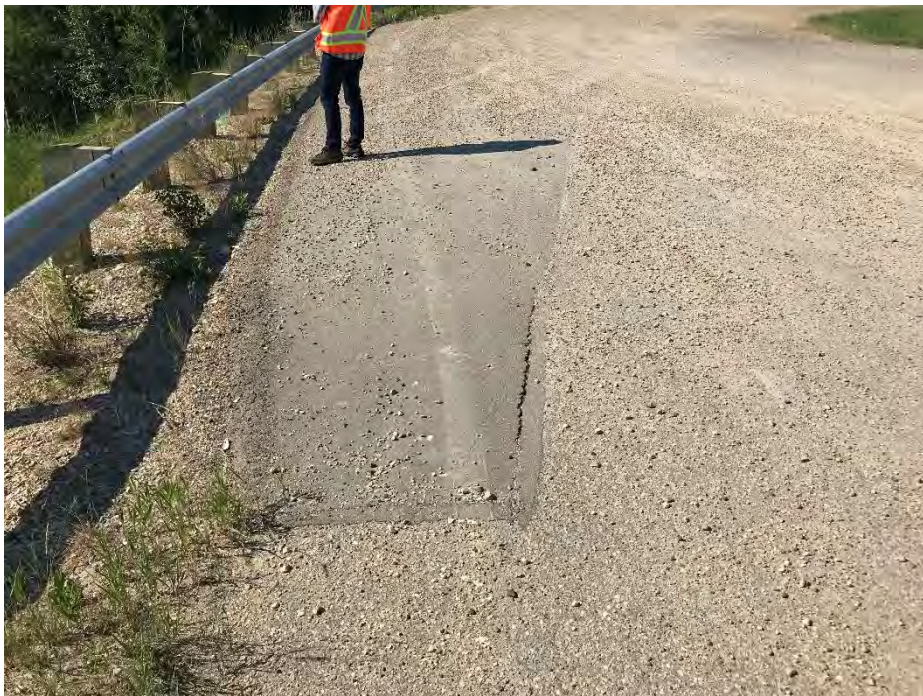
Photo 4: Separation of new and old pavement west of pile wall. Looking south.
