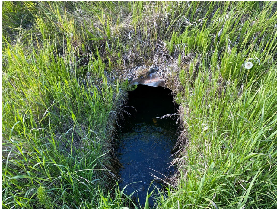
Photo 8: Water ponded in sunken culvert outlet in ditch east of private access, north side of highway. Looking south.
