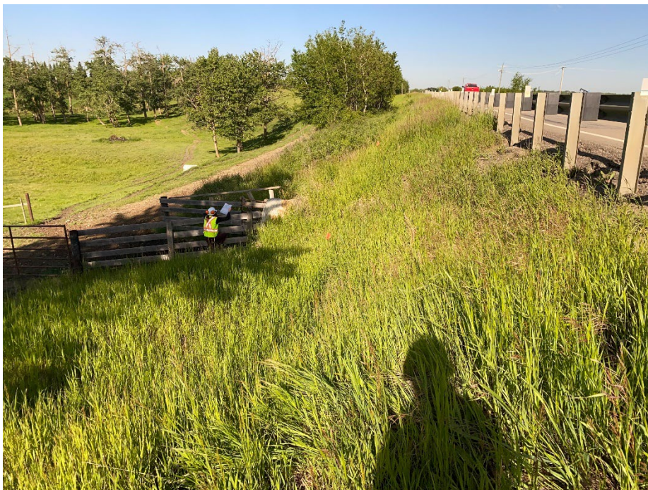
Photo 2: Slump across cattlepass culvert. Looking west
