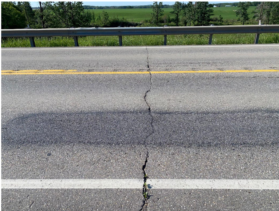
Photo 6: Transverse pavement crack above eastern scarp. Looking south.
