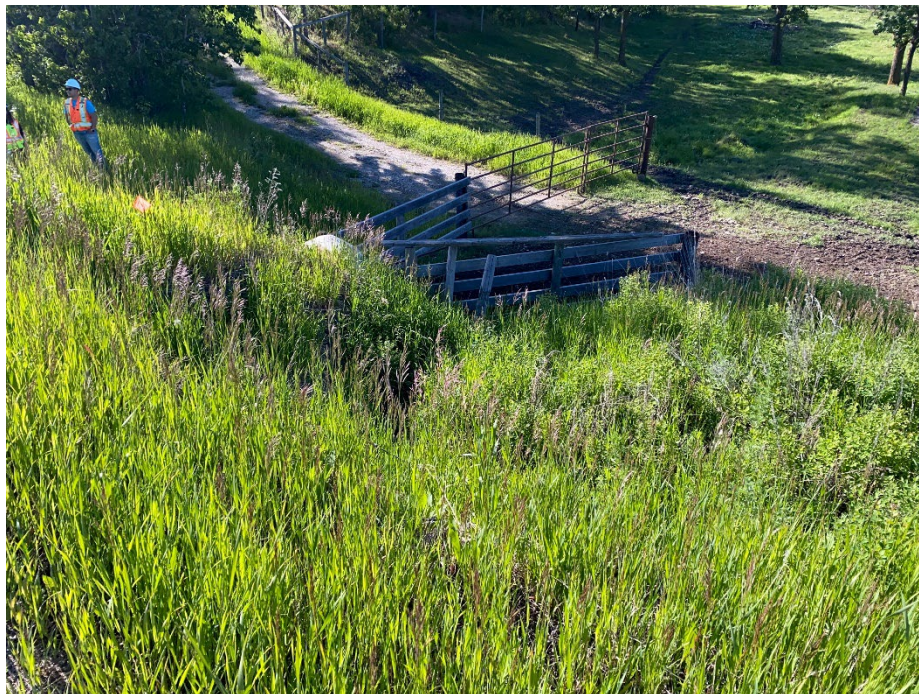
Photo 4: West slump next to culvert entrance. Looking southeast.
