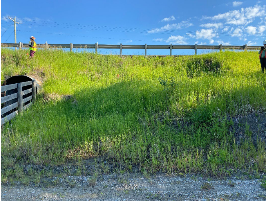
Photo 1: Slump on east side of culvert. Possible regraded area on east side of culvert, well vegetated. Looking north.
