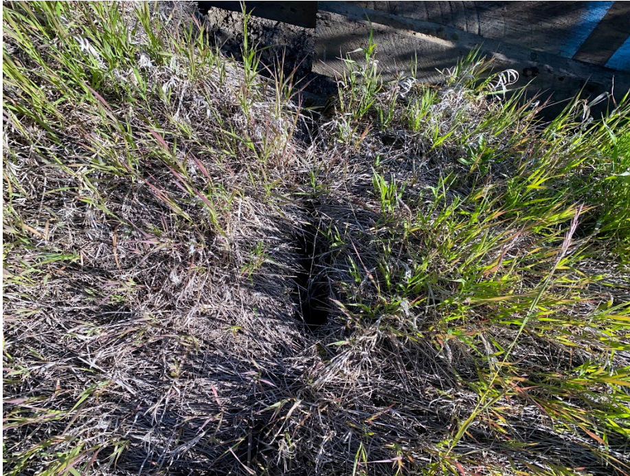
Photo 7: Ground crack along centreline of cattlepass culvert at north end. Looking northwest.
