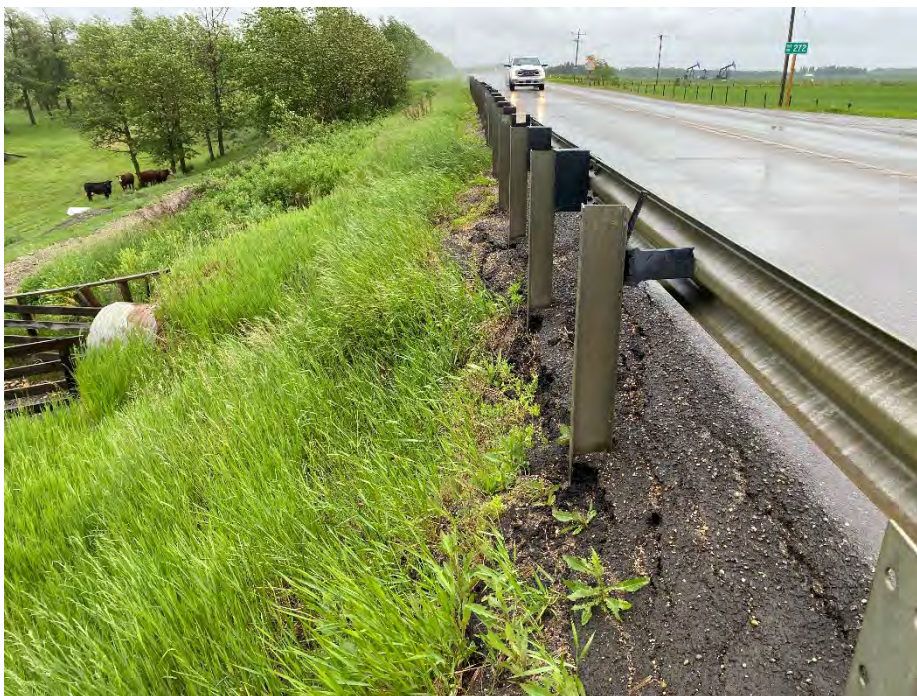
Photo 2: Slump across cattlepass culvert. Looking northwest
