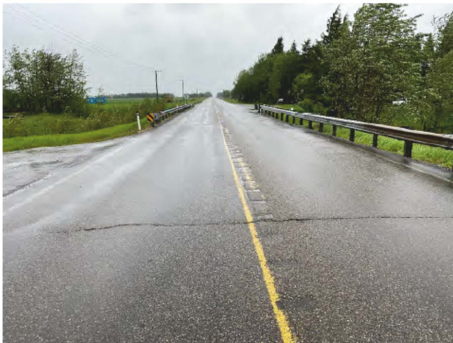
Photo 6: Highway surface at slump location. Looking east.
