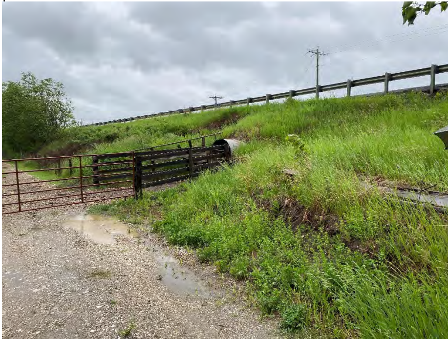
Photo 1: Slump across cattlepass culvert. Looking northwest
