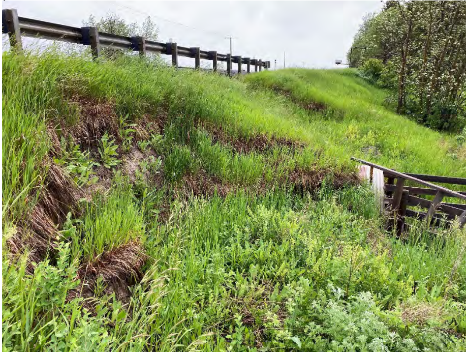
Photo 3: Scarp at west slump. Looking east.
