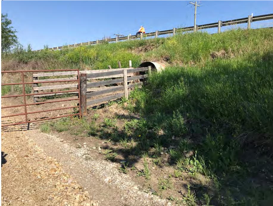
Photo 1: Slump across cattlepass culvert. Looking northwest
