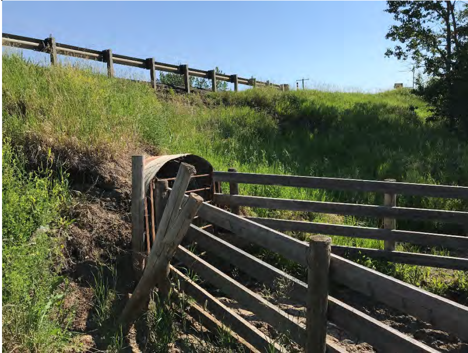
Photo 5: Fresh scarp about 1 m high adjacent at south end of cattlepass culvert. New wooden posts significantly leaning. Looking northeast.
