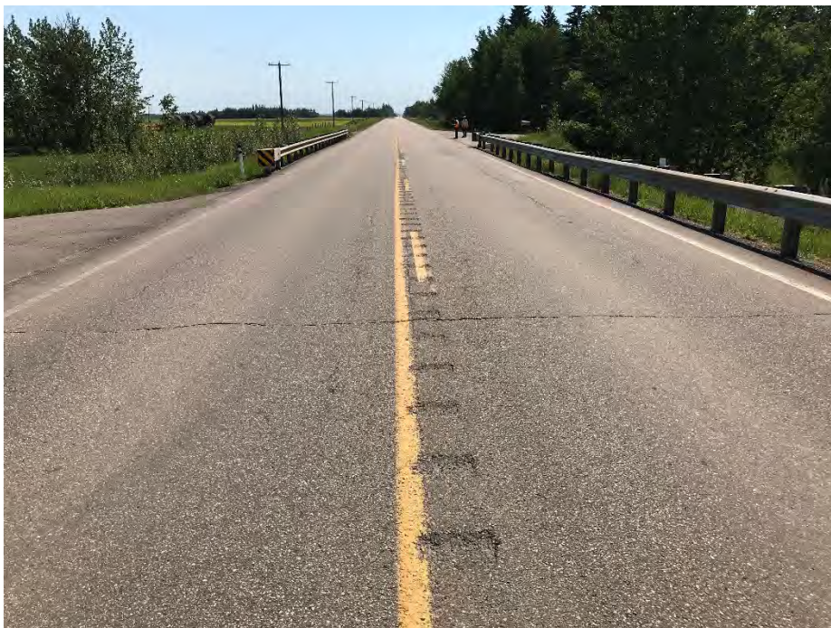
Photo 6: Highway surface at slump location. Looking east.
