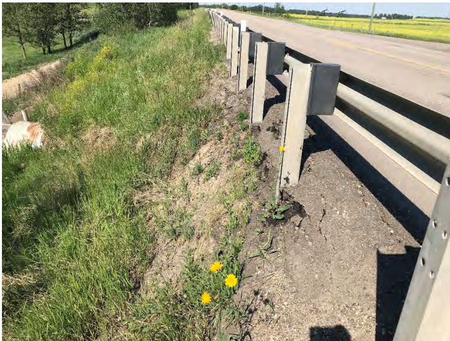
Photo 2: Slump across cattlepass culvert. Looking northwest
