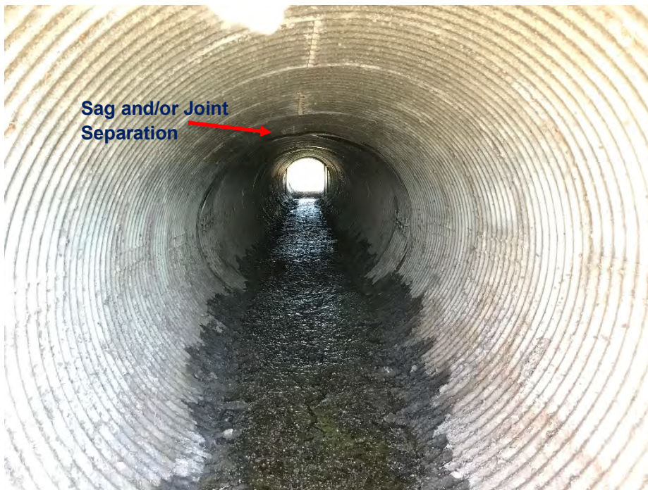
Photo 4: Sag and/or separation at south end. Looking east.
