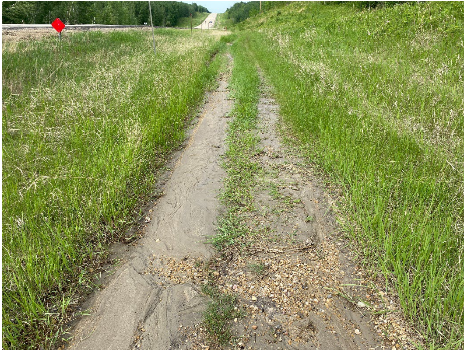
Photo 3: Signs of flowing water and sedimentation in wheel tracks on east side of highway, south from backslope slump #3. Looking north.
