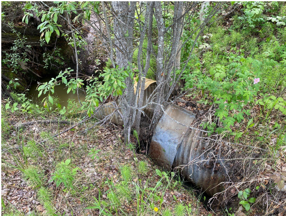
Photo 4: Separation at culvert inlet. Looking southwest.
