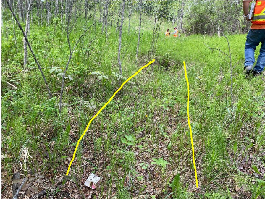
Photo 5: Subsidence along culvert alignment. Looking north.
