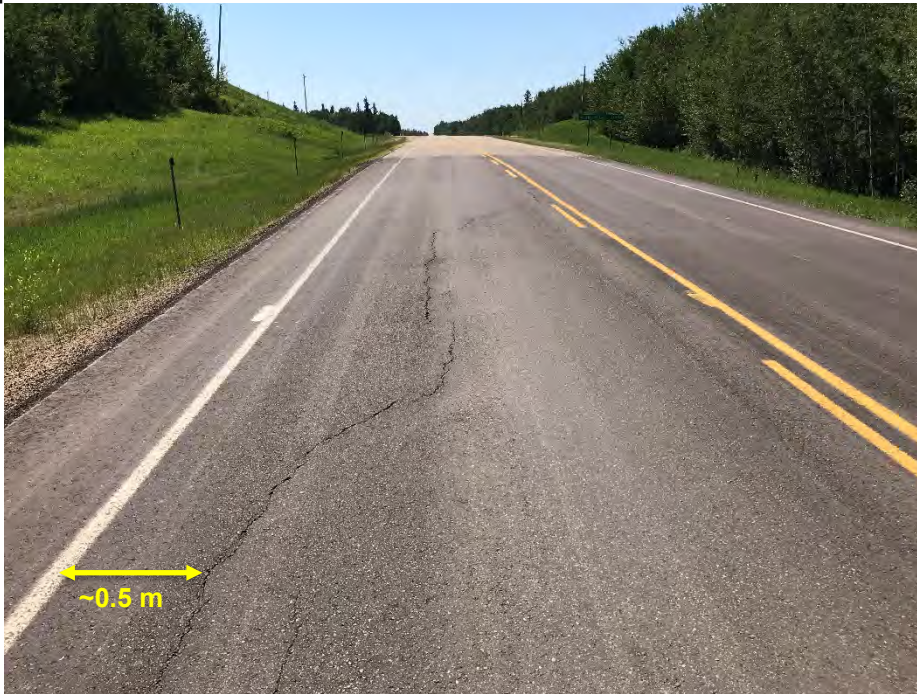
Photo 1: Pavement cracks reflecting through 2017 patch. Looking south.
