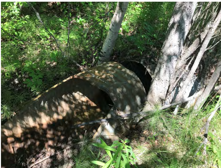
Photo 4: Separation at culvert inlet. Looking north.
