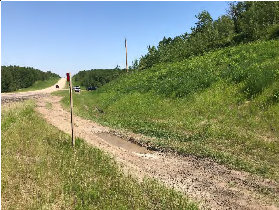
Photo 3: Ponding in wheel rut at toe of backslope slump #3. Looking north.
