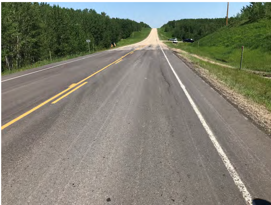
Photo 2: Pavement cracks reflecting through 2017 patch. Looking north.
