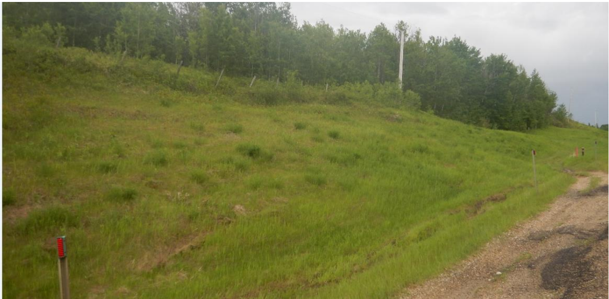
Photo No. 2 – Looking south at slump No.3 located within the limits of the landslide; the toe of the slump is encroaching in the ditch and is partially restraining ditch flow
