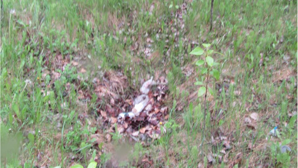
Photo No. 8 – Existing manhole, located to the west side of the highway within the bush, is partially covered with grass and leaves; water still flows into the manhole
