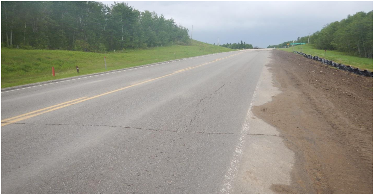
Photo No. 5a – Looking south at a reflective open longitudinal crack on the highway SBL near the middle of the landslide
