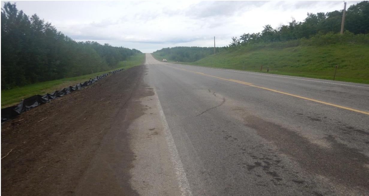
Photo No. 5c – Looking north at a reflective open diagonal at the southern flank of the landslide
