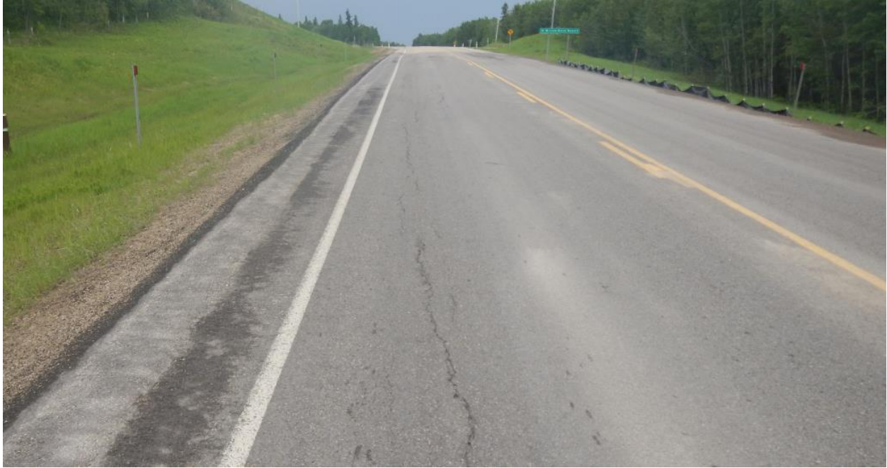
Photo No. 5 – Looking south at a reflective open longitudinal crack near the north flank of the landslide and a sharp drop off on the east side of the highway (NBL)
