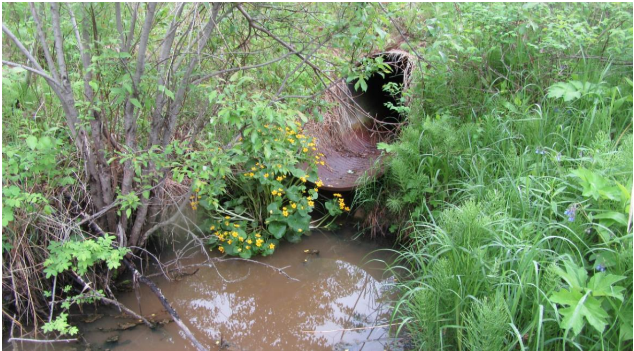
Photo No. 9 – Water flows under the culvert outlet
