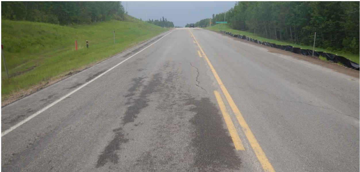
Photo No. 4 – Reflective open longitudinal crack near the north flank of the landslide
