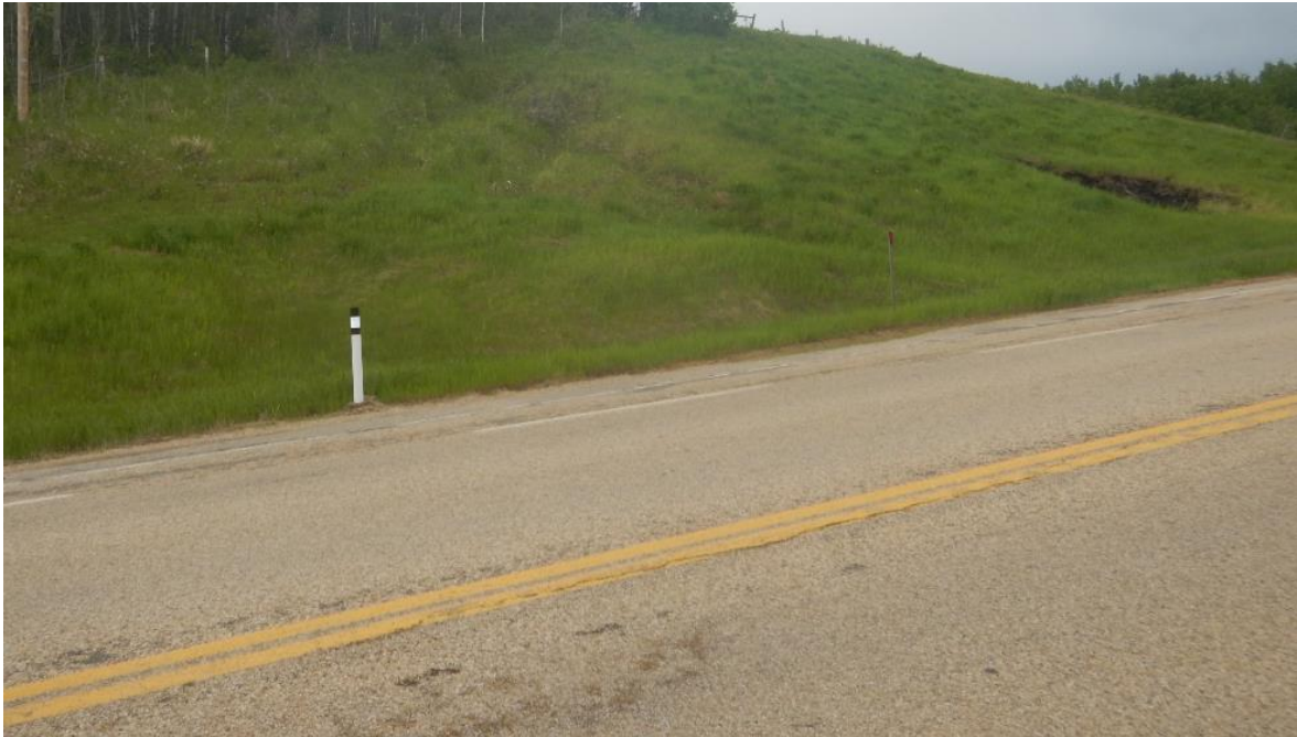
Photo No. 1 – Looking southeast at backslope slump No. 1 located to the south of the landslide area
