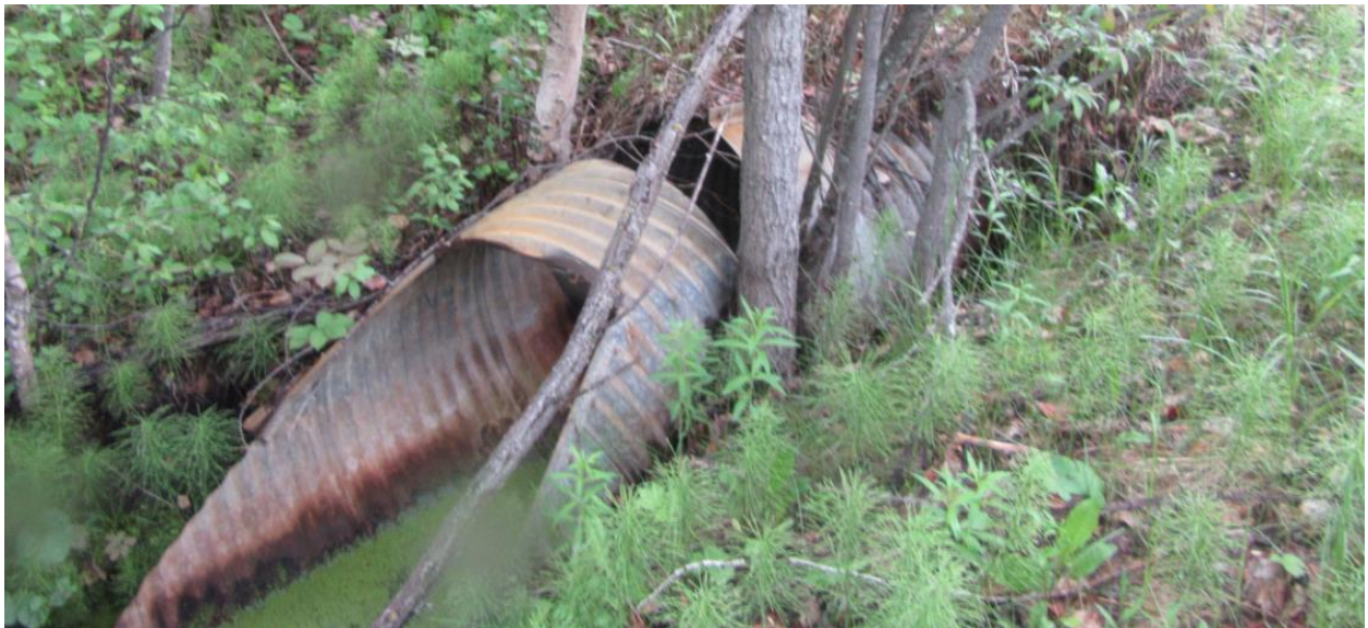
Photo No. 7 – Looking north at the separated culvert inlet
