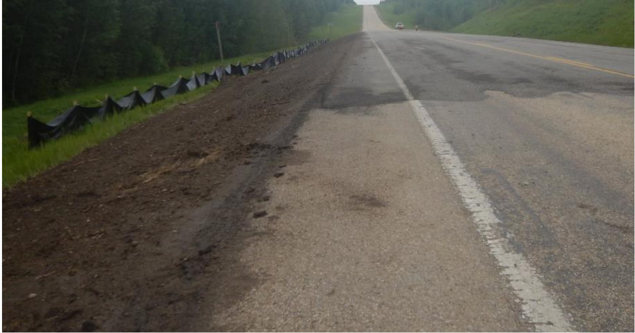
Photo No. 3 – Clay wedge placed by AT along the west side slope of the highway to eliminate previous sharp drop off (looking north)
