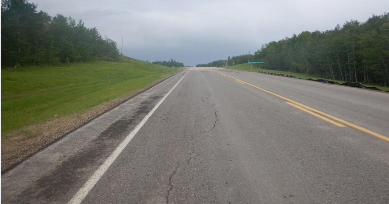
Photo No. 5b – Looking south at a reflective open longitudinal crack on the highway NBL near the middle of the landslide
