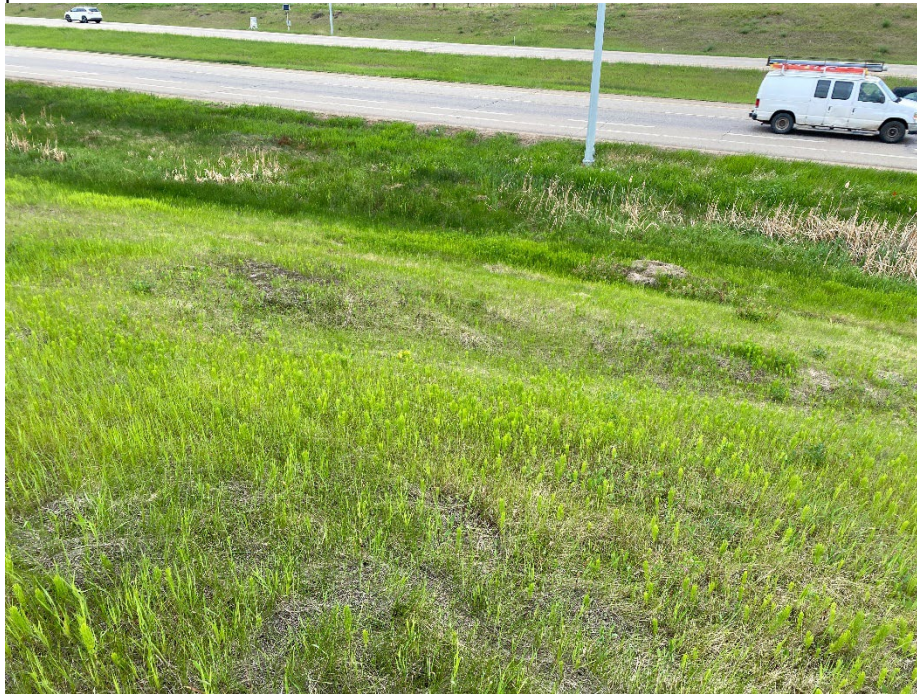
Photo 5: View of west extent of slump looking downslope. Facing northwest.
