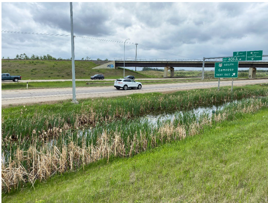
Photo 6: Water ponding in ditch with long grasses and reeds. Looking northeast.
