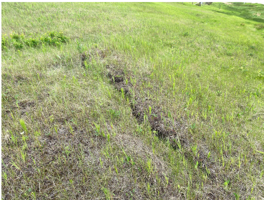
Photo 4: Ground crack (1.8 m long) running vertically across the slope, downslope from scarps. Looking west.
