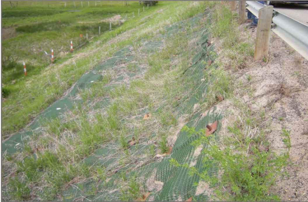
Photo 1: Repaired sideslope requires topsoil and seeding
