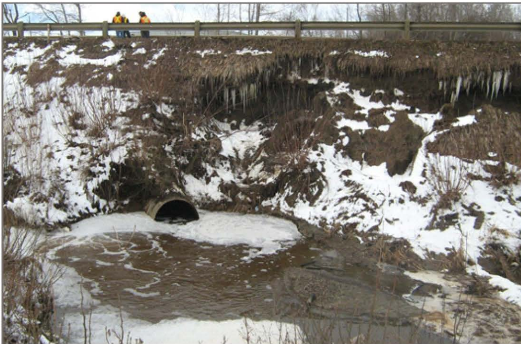
Photo 4a: Extent of slope failure on downstream side of blocked culvert. Facing northwest.
