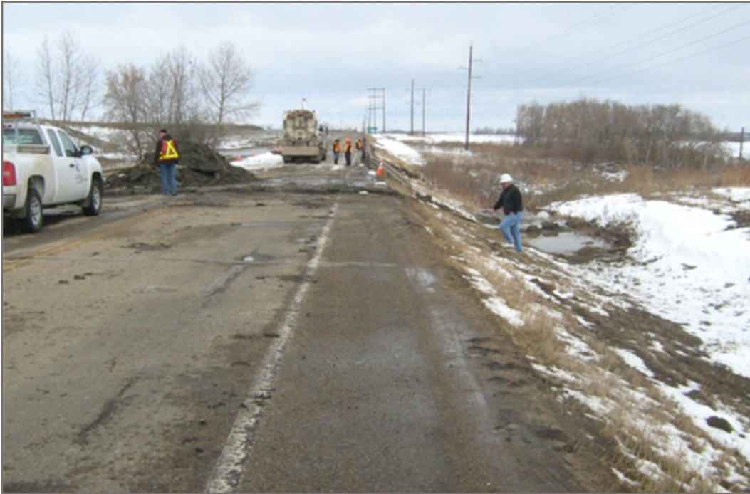
Photo 1: Hwy 825 washout due to blocked culvert. Facing northeast.
