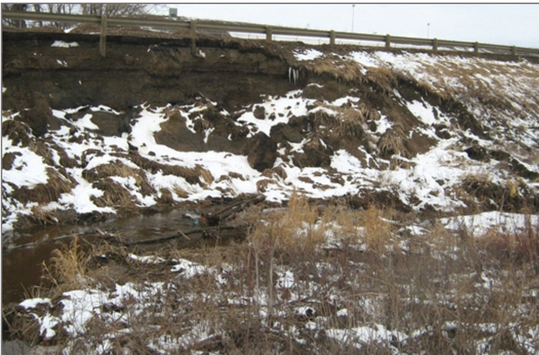
Photo 4c: Extent of slope failure on downstream side of blocked culvert (continued). Facing northwest.
