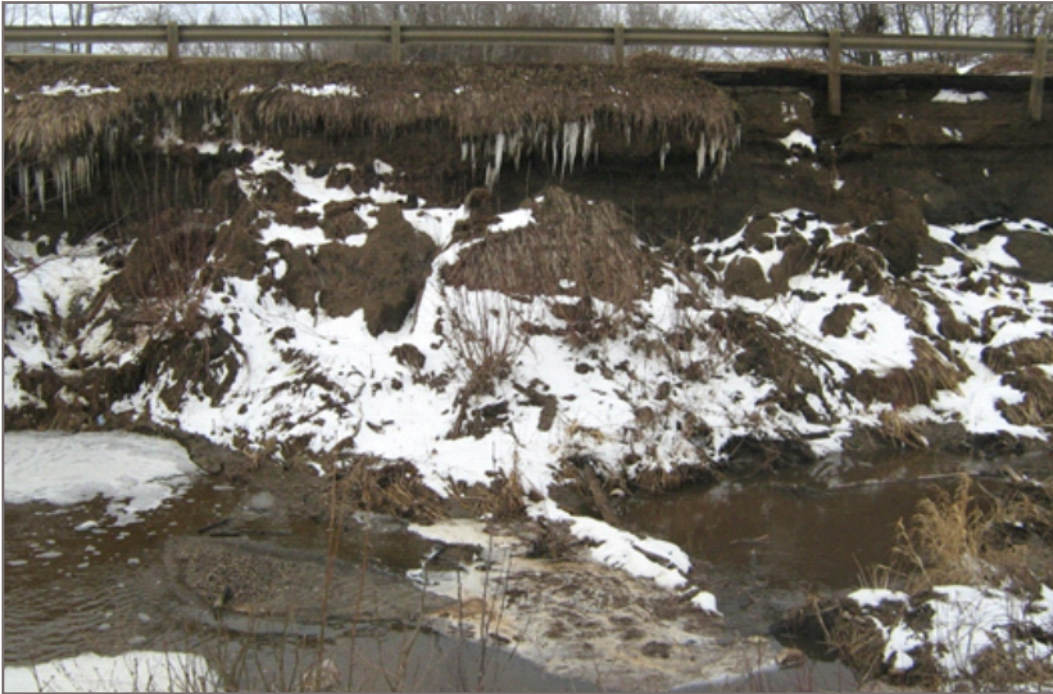
Photo 4b: Extent of slope failure on downstream side of blocked culvert (continued). Facing northwest.
