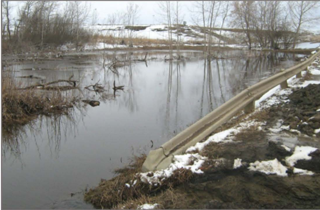
Photo 3: Flooding on upstream side of blocked culvert of Hwy 825. Facing northeast.
