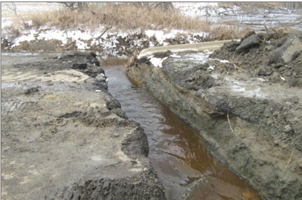
Photo 2: Trench across Hwy 825 promoting drainage due to blocked culvert. Facing northwest.
