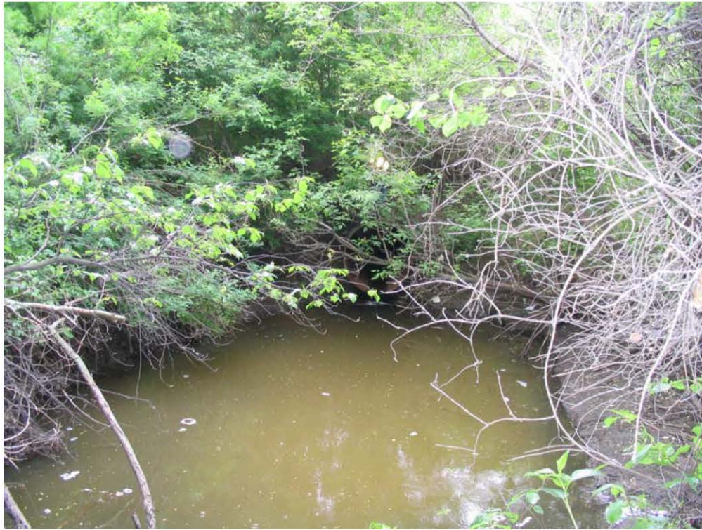
Photo 3 - Scour at the culvert outlet, June 7, 2006.
