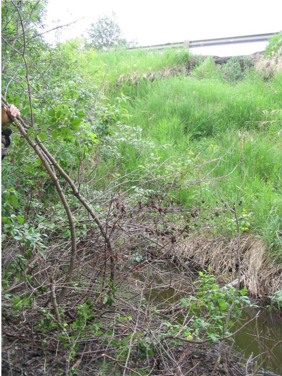
Photo 5 - Looking west at toe of slide zone, June 7, 2006.
