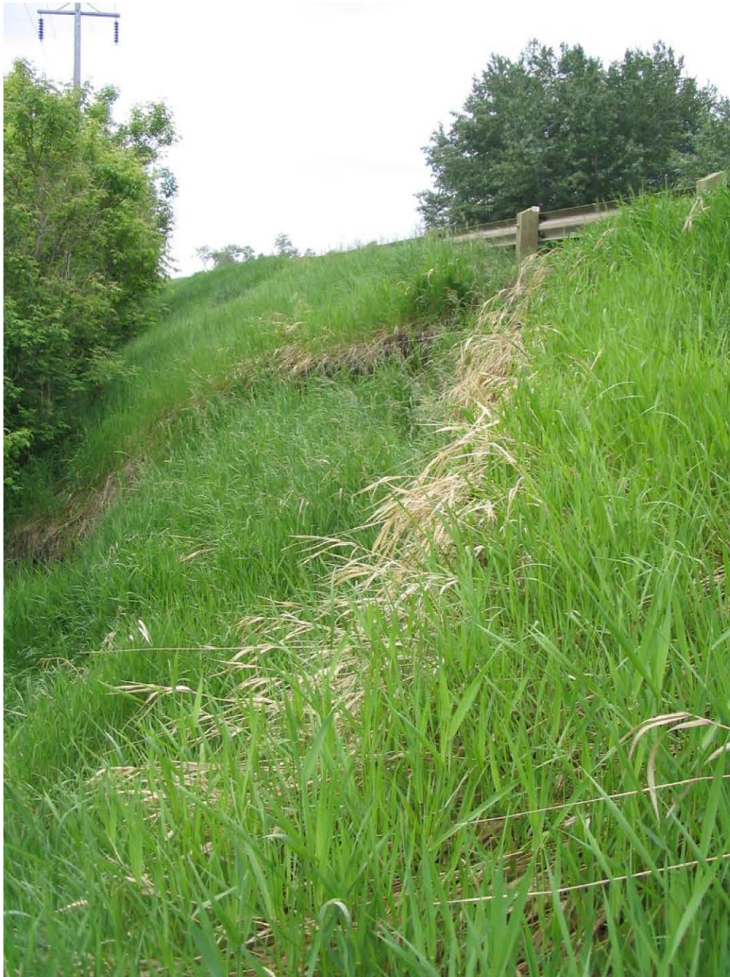
Photo 6 - Scarp to the east of the creek, June 7, 2006.
