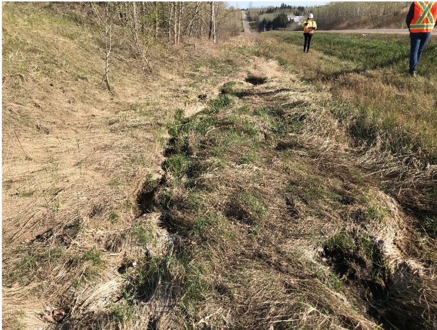
Photo 3: Erosion gullies along west ditch. Looking north.
