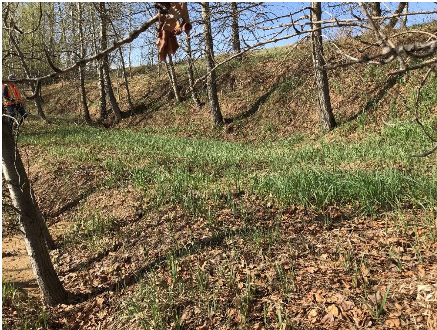
Photo 4: Well vegetated graben. No fresh cracking observed. Looking southwest.
