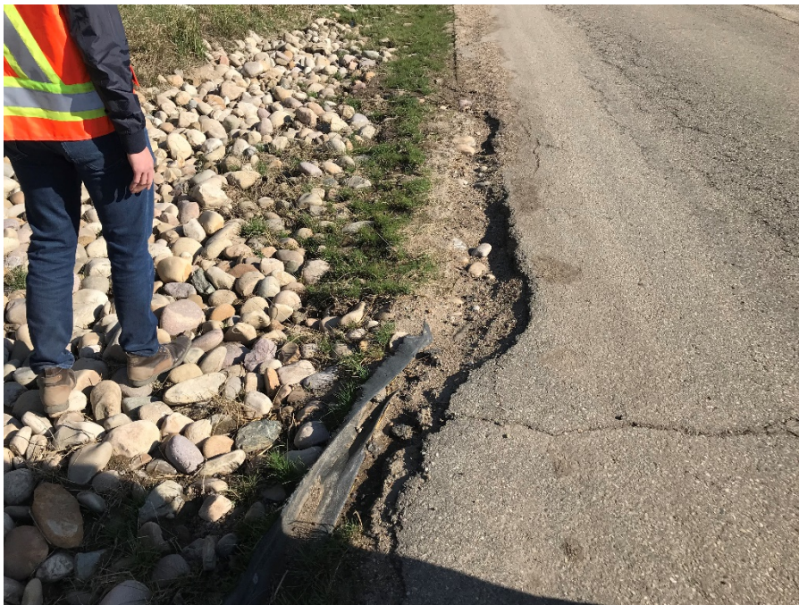
Photo 2: Collapsed pavement shoulder along rip rap approximately 200 mm wide. Looking north.
