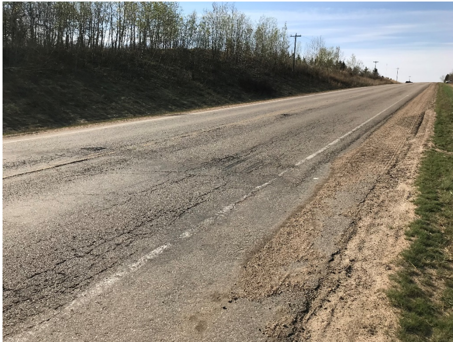
Photo 1: Patch of pavement distress approximately 10 m north of rip rap. Looking southeast.
