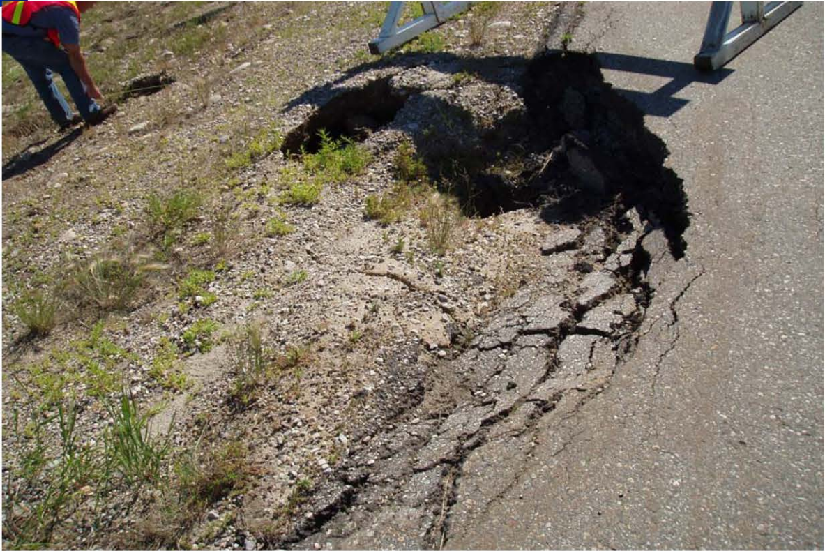
PHOTO 3: Exit hole of piping tunnel No. 3, penetrating into the pavement.
