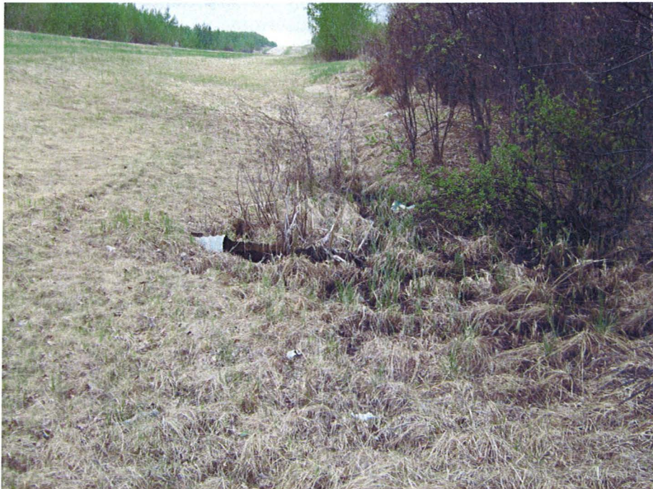
Blocked culvert and poor ditch drainage along west ditch
