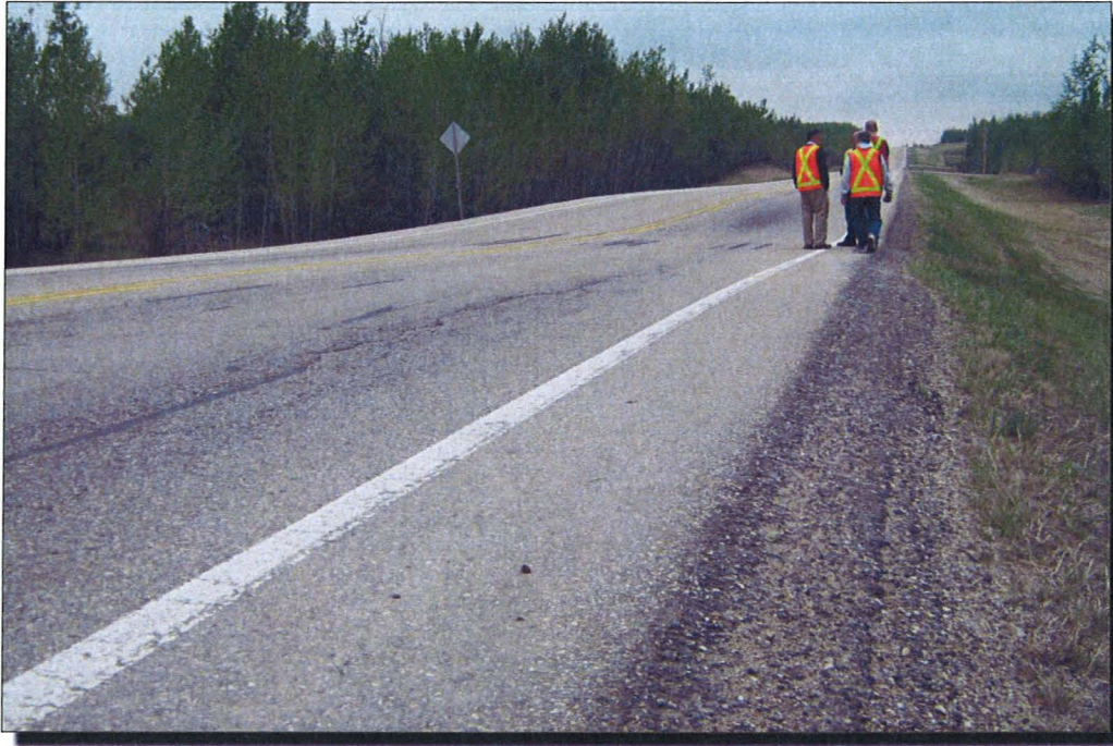
Photo 1 Pavement dip site, facing north
