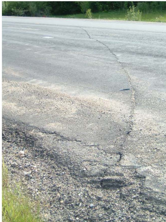
Photo 2. Main crack reappears through the new overlaid asphalt patch (2005).
