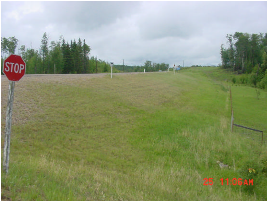
PHOTO NC16-1 LOOKING SOUTHEAST AT EMBANKMENT REPAIR AREA CULVERT OUTLET IN BOTTOM RIGHT CORNER
