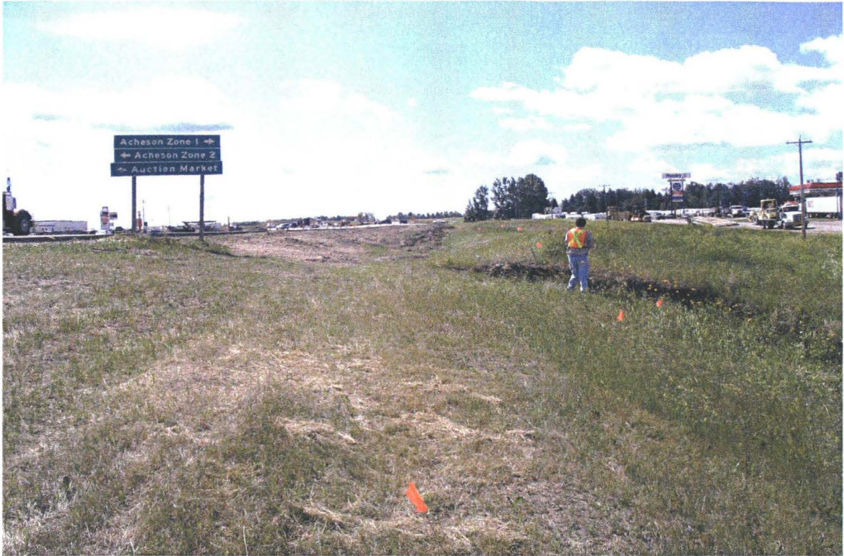
PHOTO 1: Looking south at the location of ditch erosion. Grading associated with the construction of a turning lane is visible further to the south.
