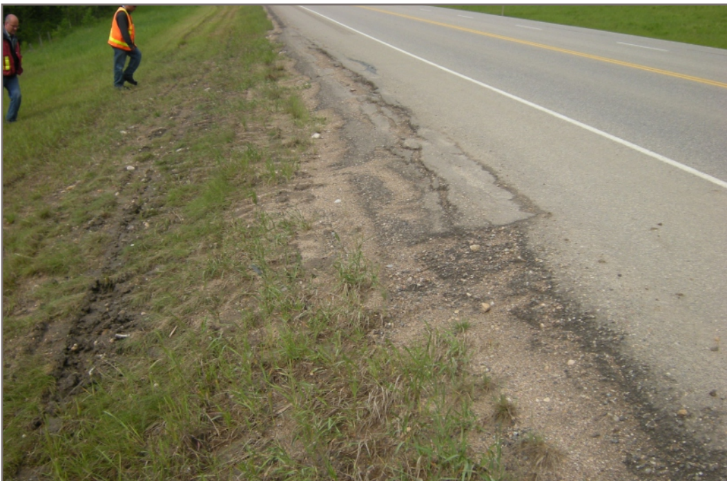
Photo 2: Cracking at edge of pavement at Site B
