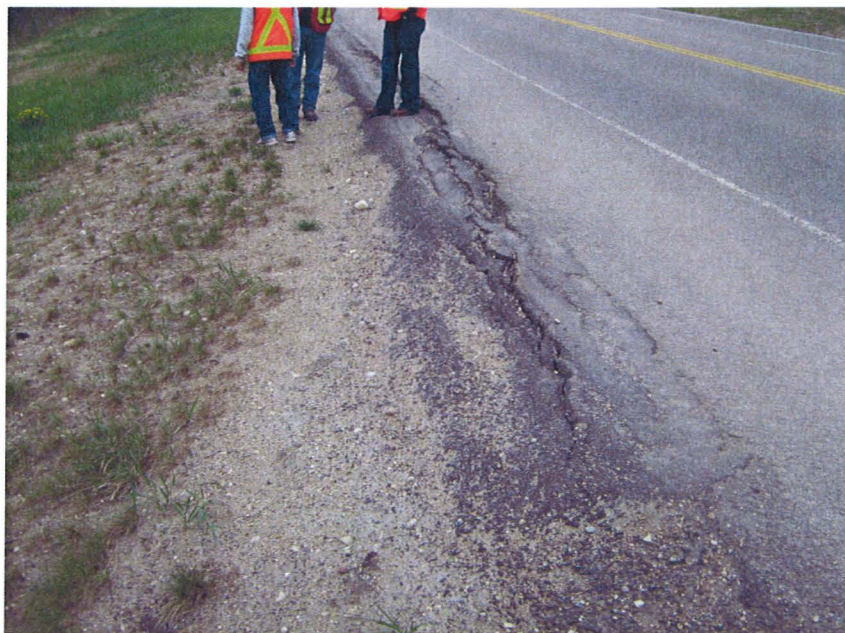
Cracking along eastbound lane and top of repaired area. Poor vegetation growth along top of embankment.
