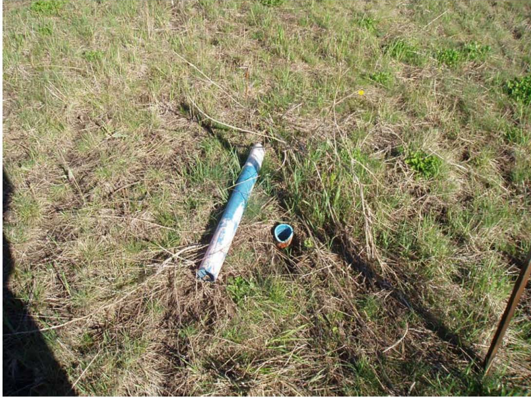
Photo 4 – SI01-2A – Stick up broken and pipe is bent at 0.75m depth.
