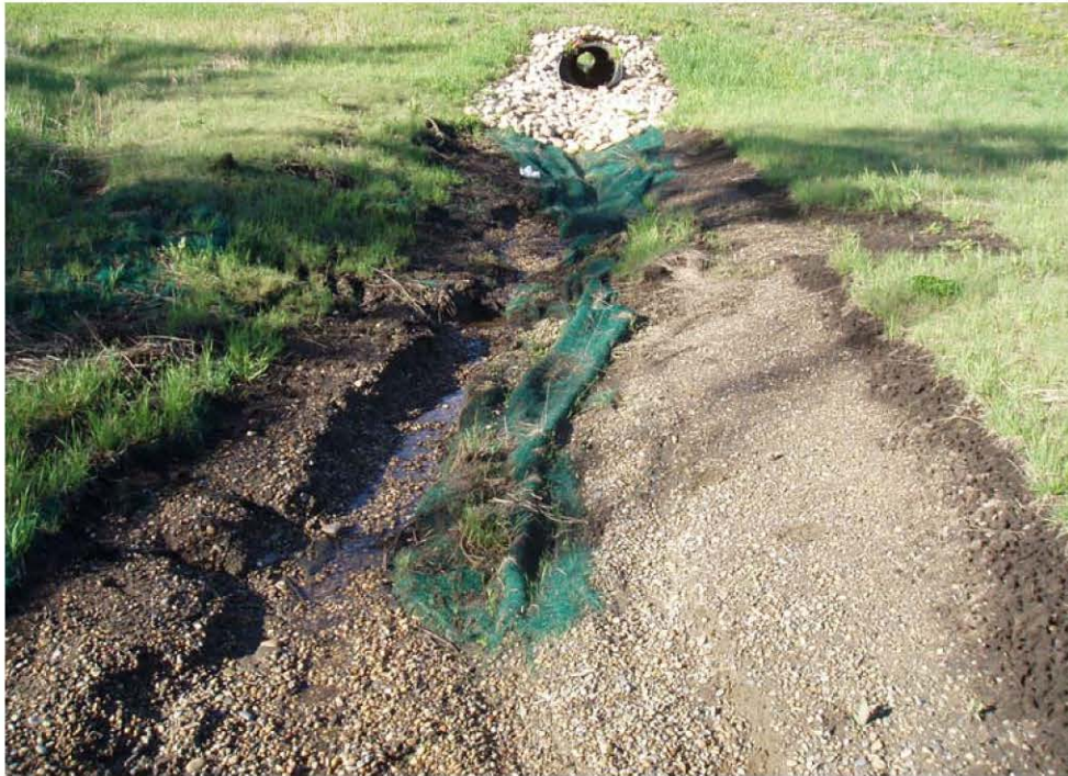
Photo 1. Culvert outlet scour
