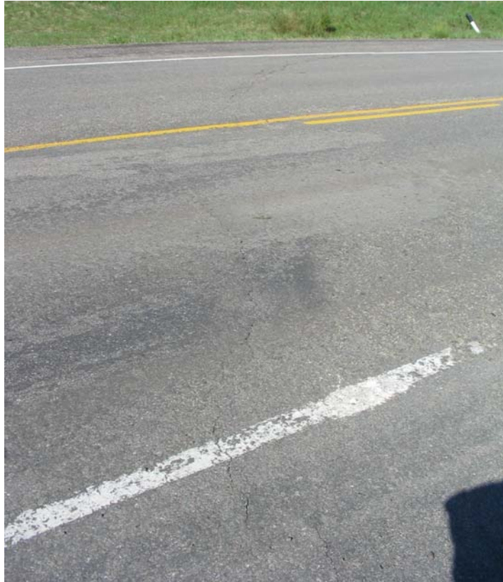
Photo 1. New crack at the east flank.
