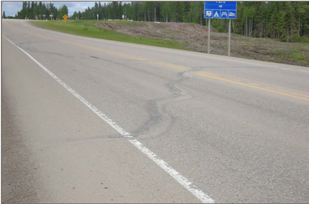
Photo 1: Sealed crack and dip in pavement overlay
