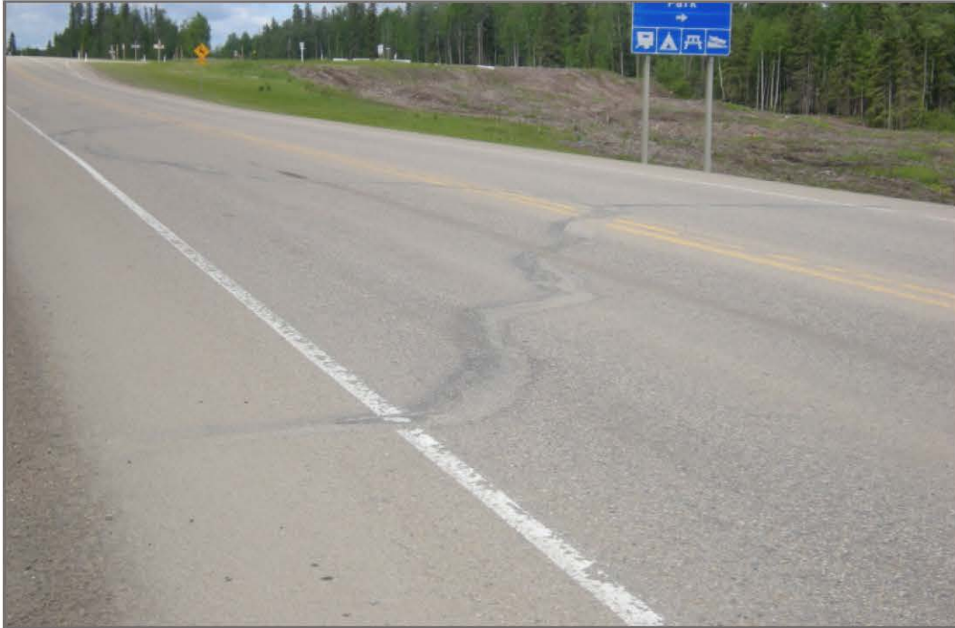
Photo 1: Sealed crack and dip in pavement overlay
