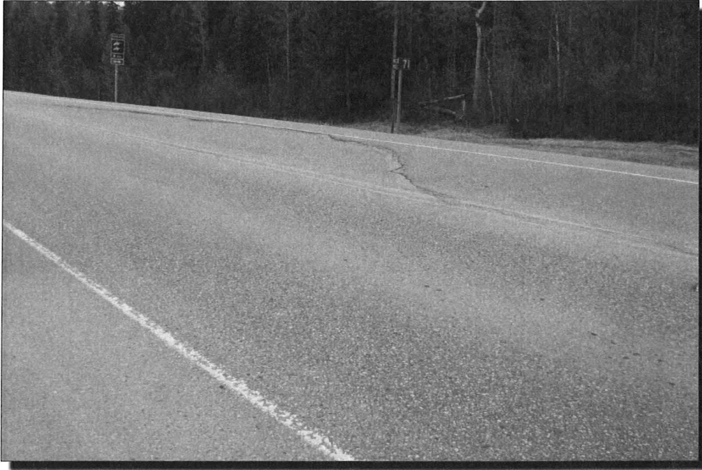
Photo 1 Crack and dip in pavement on eastbound lane
