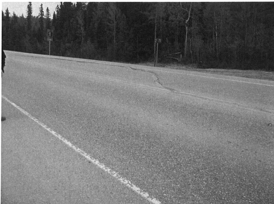
Evidence of cracking through 2004 overlay along eastbound lane
