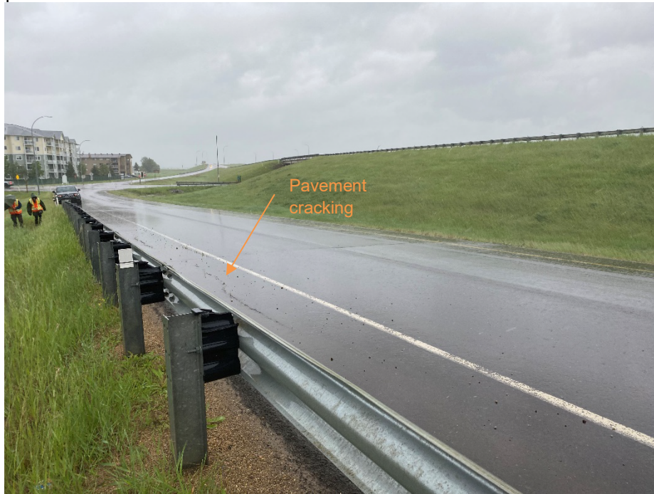
Photo 5: On-ramp to Highway 2 north bound. Cracking approx. 40 m south of south slide. Looking south.
