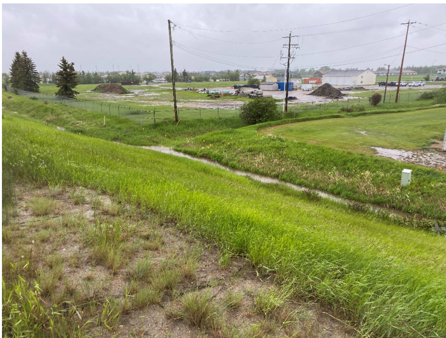
Photo 4: Road sand leading appears to be reducing vegetation at crest of embankment at south slide Facing northeast.
