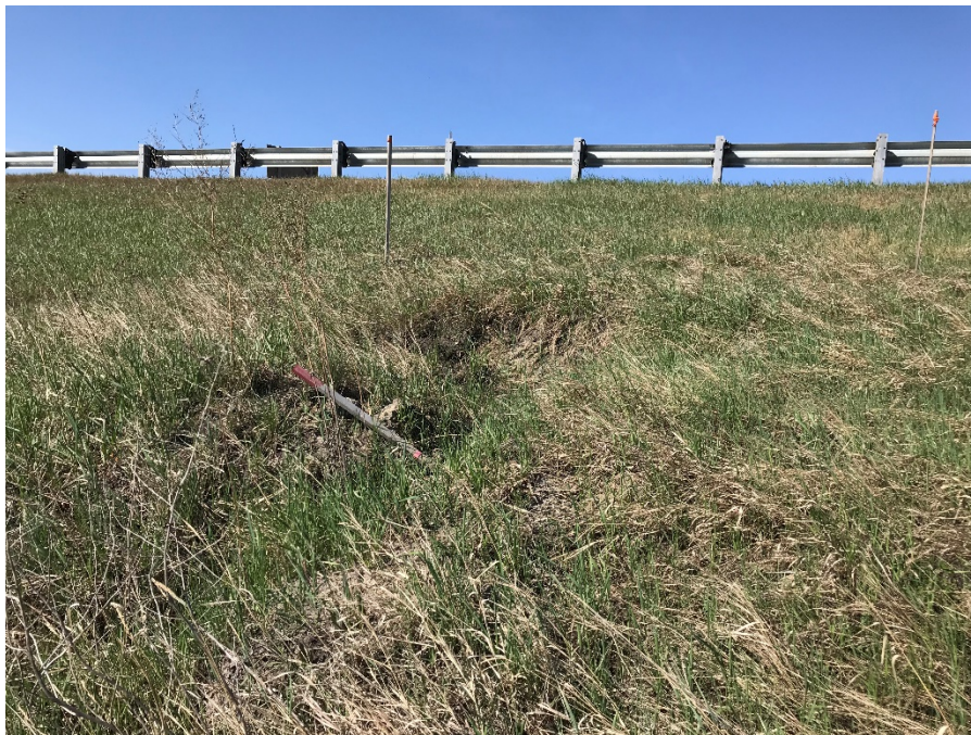
Photo 3: Slumping at previous test pit location. Looking west.
