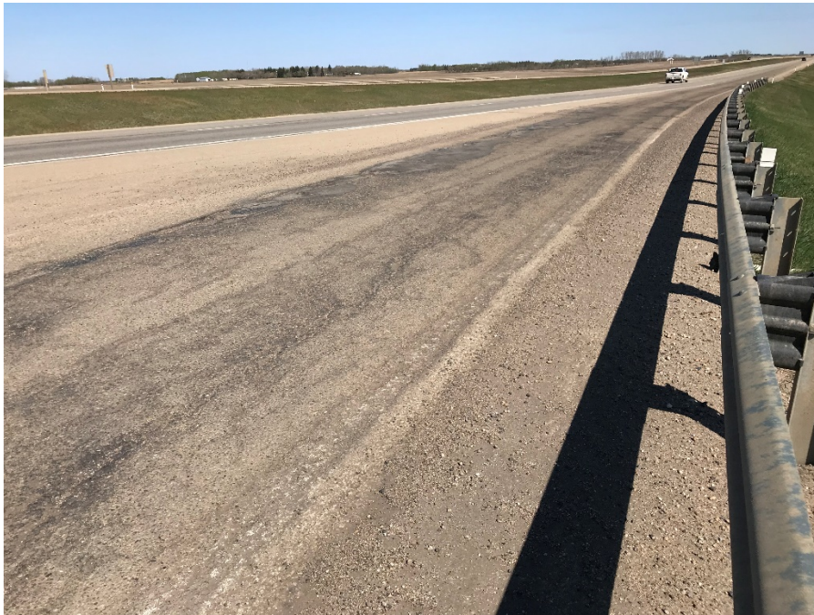
Photo 7: Highway 2 surface at north slide. Looking north.
