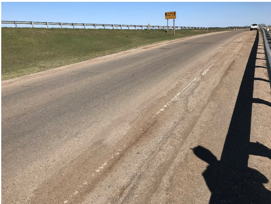
Photo 8: Highway 2 surface at south slide. Looking north.
