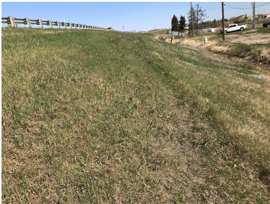
Photo 4: New ground crack at southern limits of south slump repair. Looking north.
