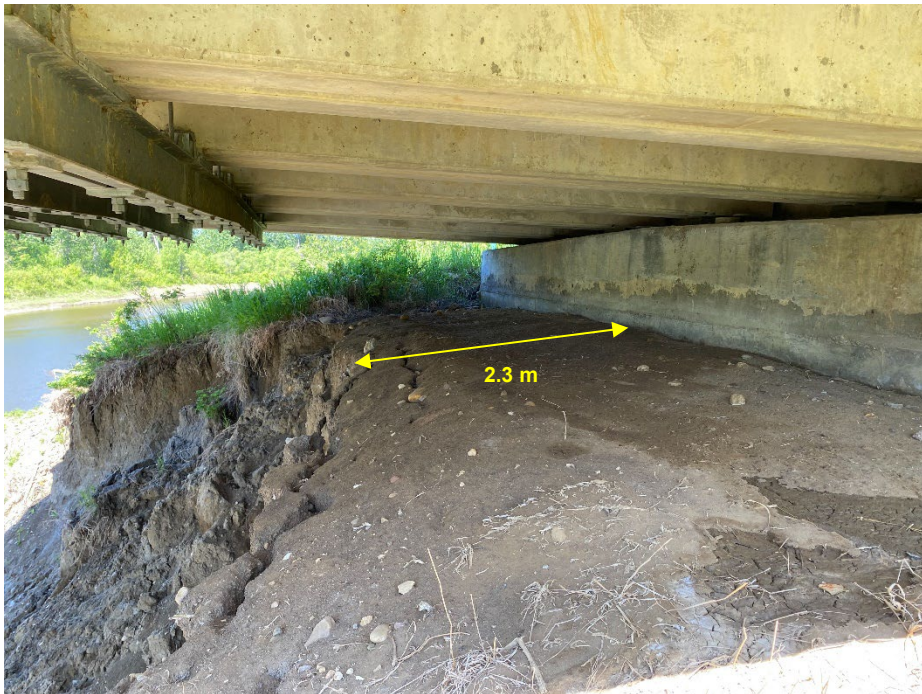
Photo 6: North abutment head slope washed away with further tension cracks. Looking northwest.
