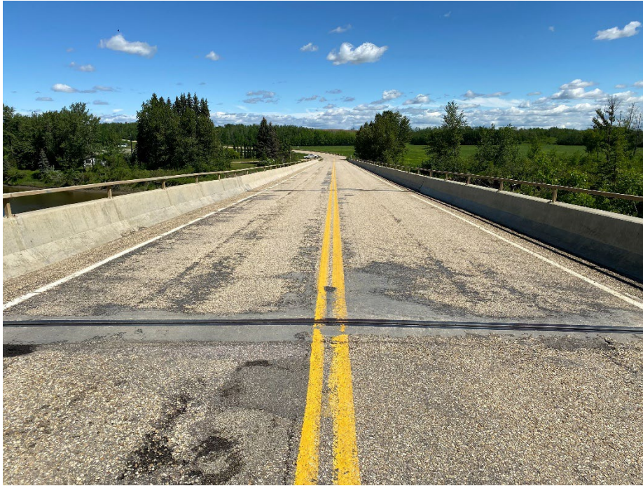
Photo 3: Highway surface at south abutment. Looking northeast.
