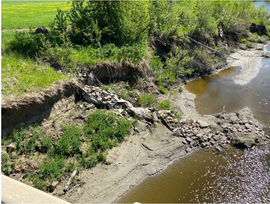
Photo 7: East extent of washout at north abutment. Note collapsed riprap channel wrapped in geotextile. Looking east.
