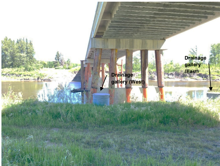
Photo 12: Saturated ground between drainage galleries and Pier 1. Looking northeast.
