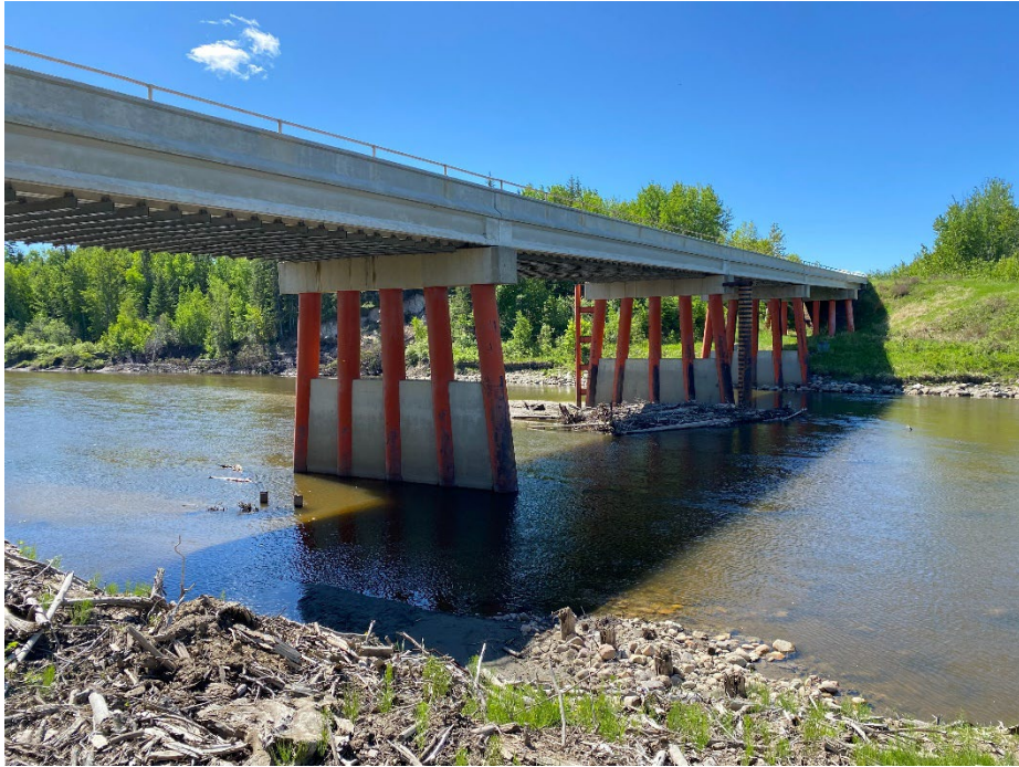
Photo 5: Majority of drift accumulation upstream under bridge removed. Looking southeast.
