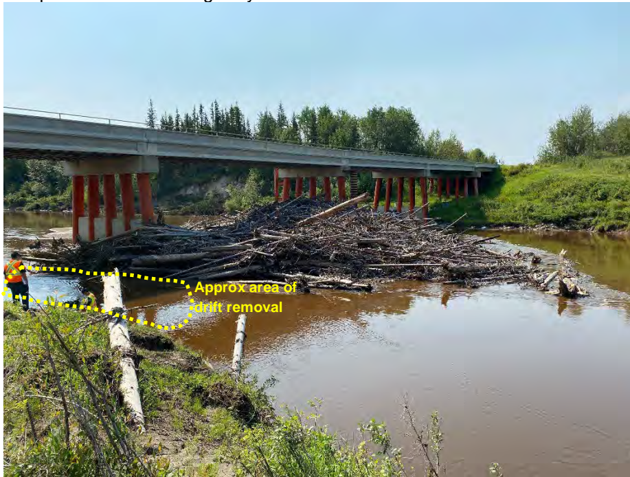
Photo 5: Drift accumulation upstream of bridge. Looking southeast.
