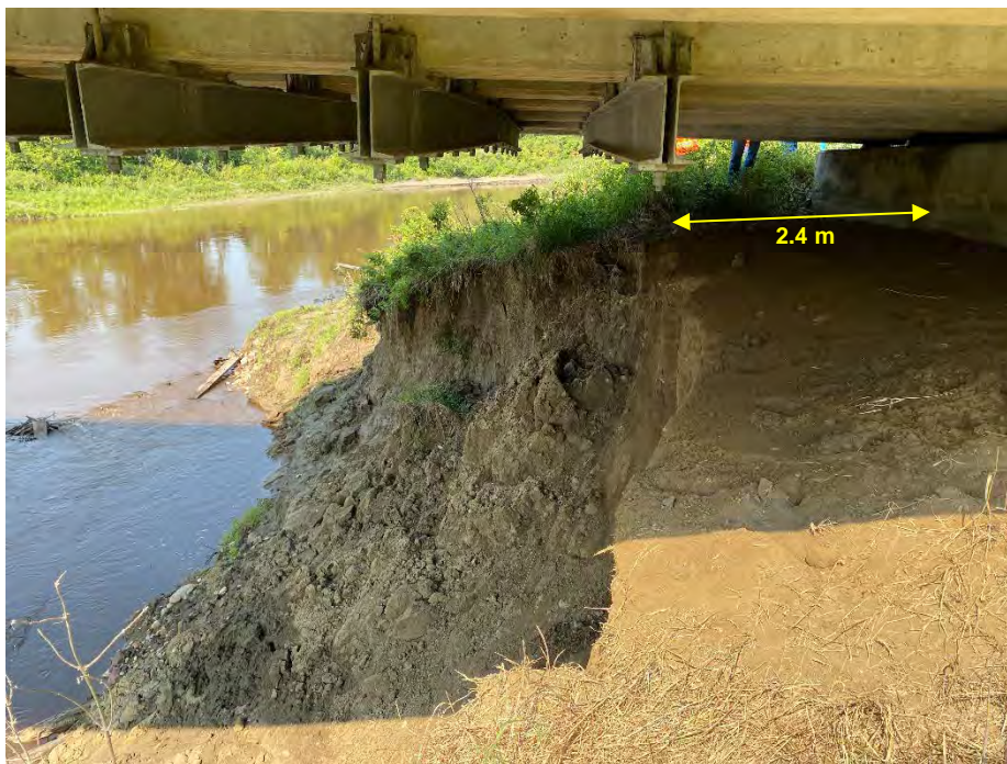
Photo 6: North abutment head slope washed away. Looking northwest.
