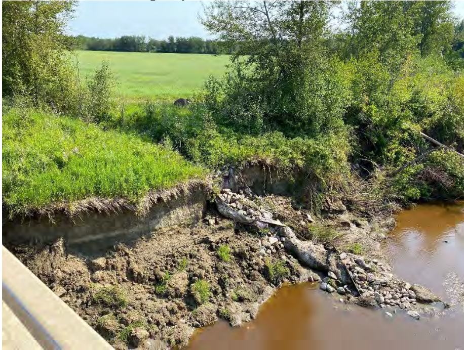
Photo 7: East extent of washout at north abutment. Note collapsed riprap channel wrapped in geotextile. Looking east.
