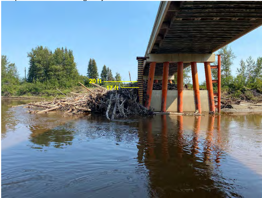
Photo 13: Drift accumulation upstream of bridge up to about 20 ft mark. River level up to 17 ft mark during flooding. Looking northeast.
