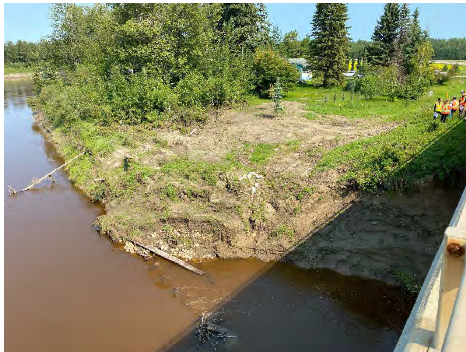
Photo 8: West extent of washout at north abutment. Looking north.
