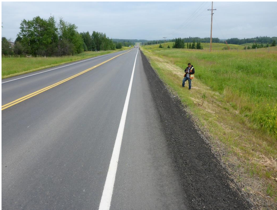
Photo 2: Steep east edge from recent overlay. Looking north.
