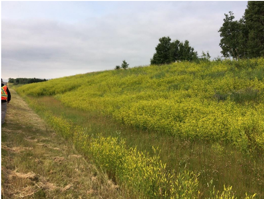
Photo 5: Grass growth over slumping hill at south end of site. Looking southwest.
