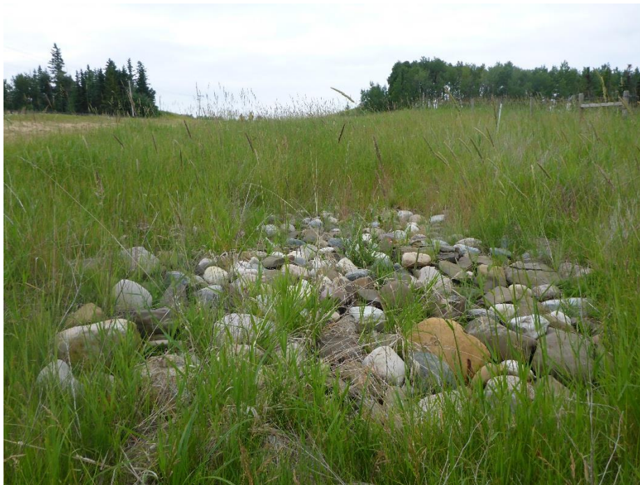
Photo 4: Culvert paralleling overhead powerline missing. Patch of riprap remains. Looking south.
