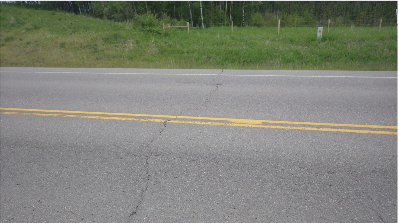
PHOTOGRAPH 5: Transverse crack at south end of site, facing west.
