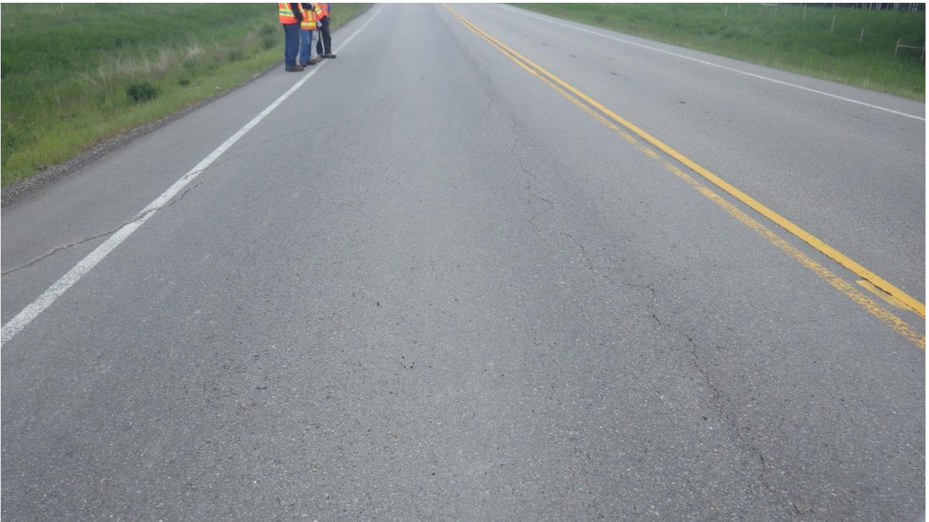
PHOTOGRAPH 3: Pavement distress near midpoint of site in northbound lane, facing south.
