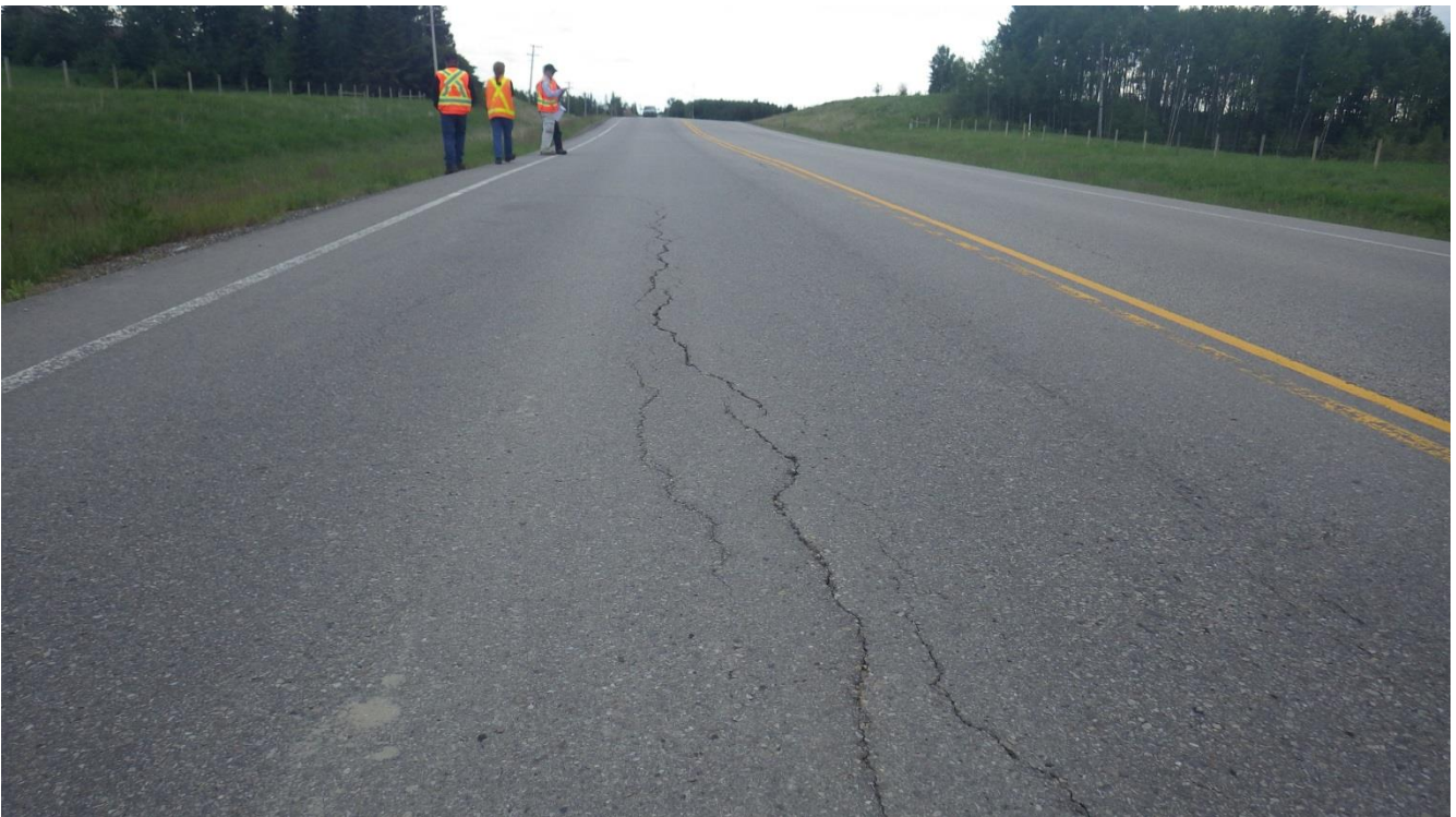
PHOTOGRAPH 4: Pavement near midpoint of site in northbound lane, facing south.
