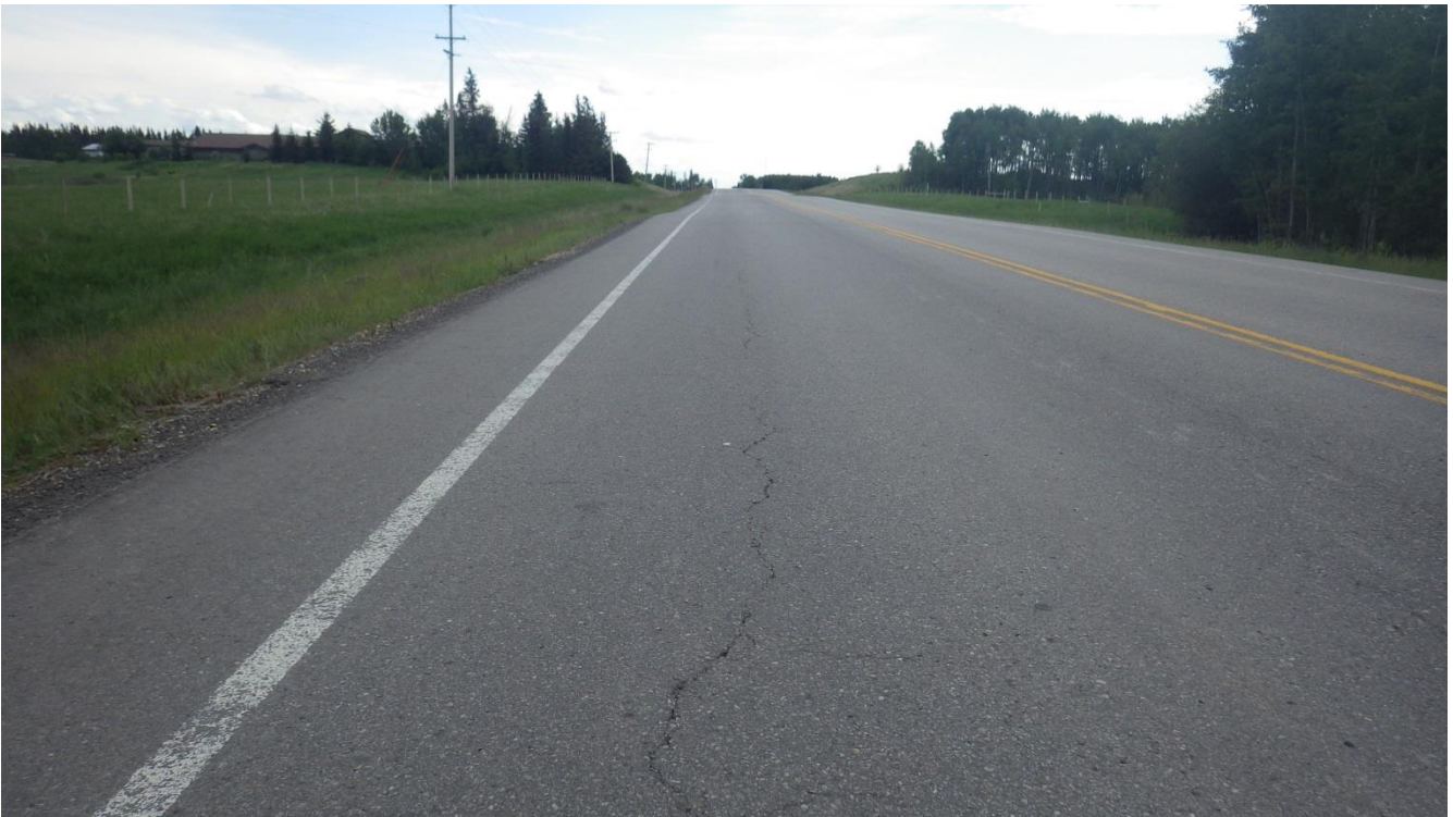
PHOTOGRAPH 1: Pavement crack at north end of site in northbound lane, facing south.
