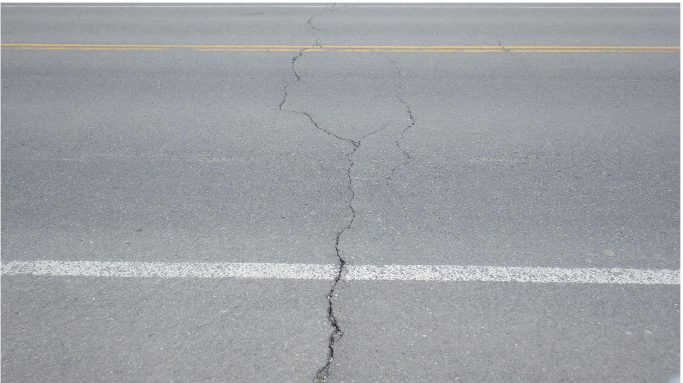
PHOTOGRAPH 2: Transverse pavement crack at north end of site, facing west.
