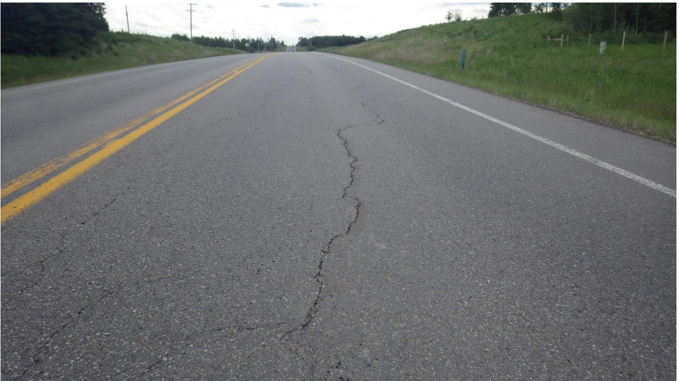
PHOTOGRAPH 6: Pavement distress at south end of site in southbound lane, facing south.
