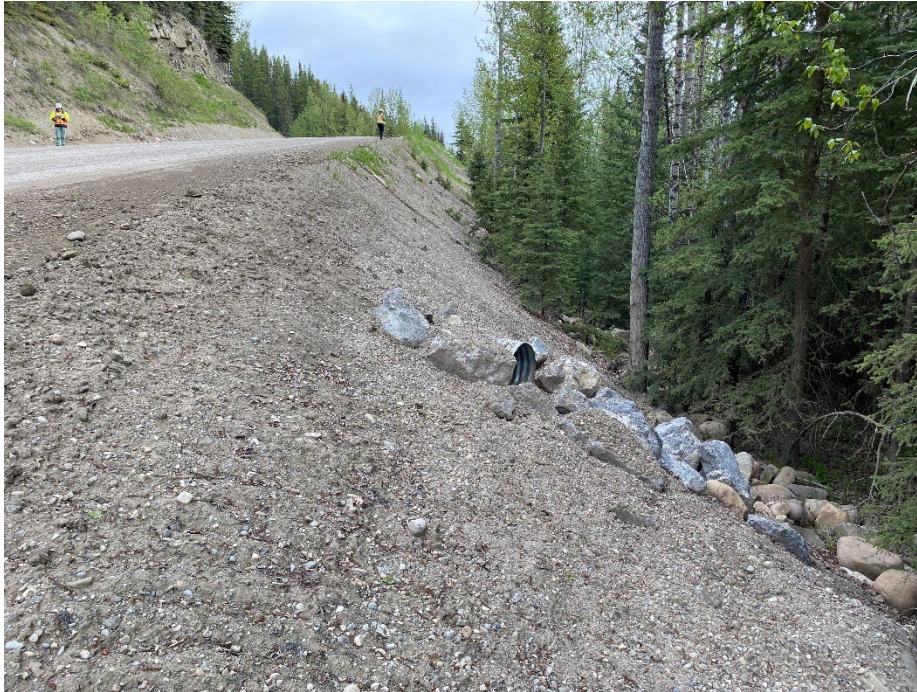
Photo 3: 600 mm diameter Culvert G installed between Culverts E and F. Outlet lined with riprap. Looking north.
