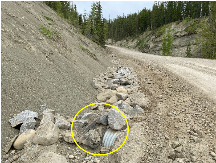
Photo 8: Culvert A inlet in SBL ditch, open and dry. Riprap lining ditch north of inlet. Looking north.
