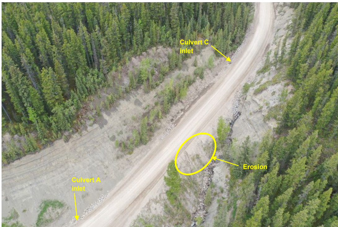
Photo 16: Overview of Highway 734 between Culverts C and A. Photo taken by drone, looking west.
