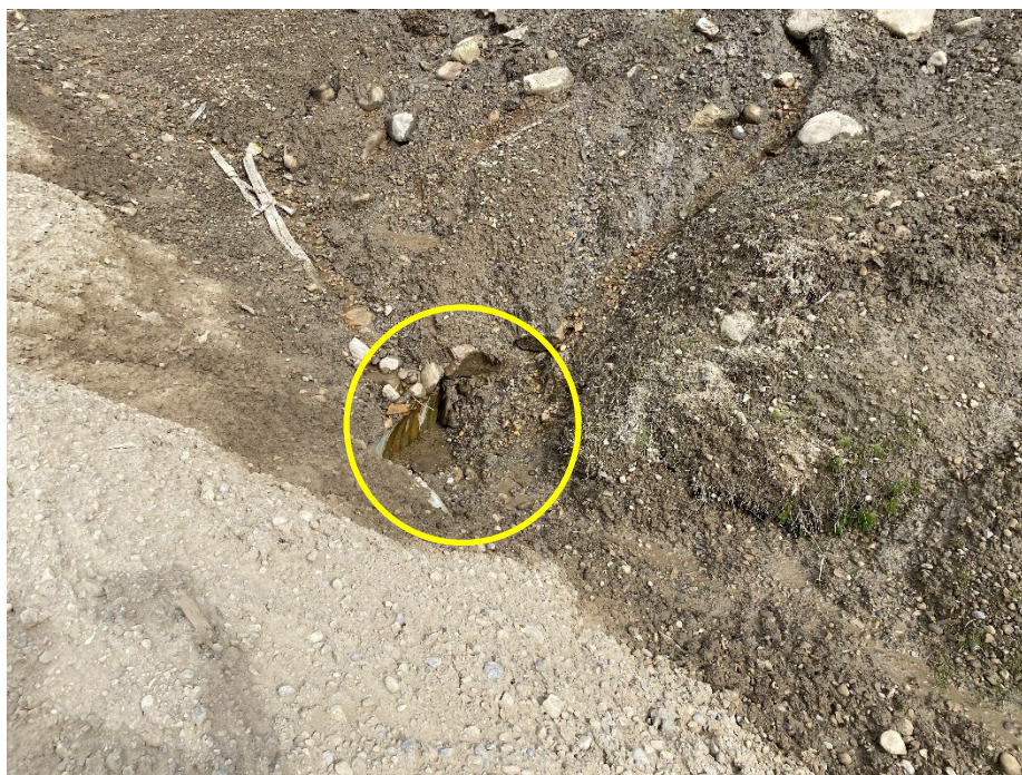
Photo 12: Inlet to Culvert H is blocked with wet material off backslope. Looking northwest.
