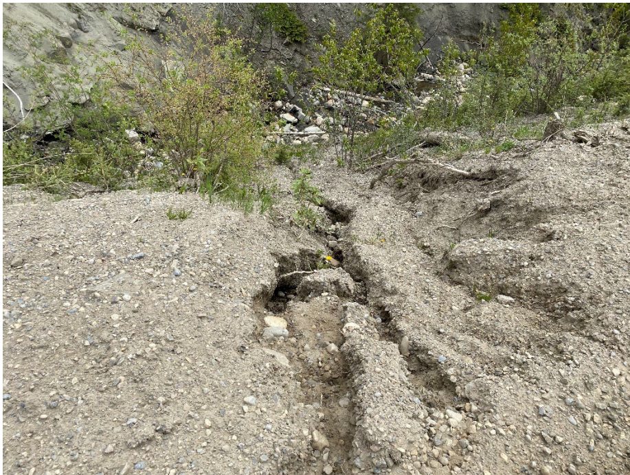
Photo 10: Erosion gully on shoulder of NBL into drainage, between Culverts A and C. Looking east.
