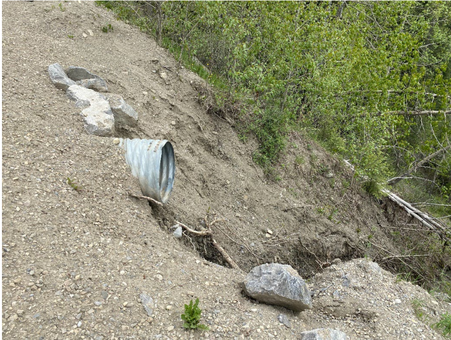
Photo 9: Overhang at Culvert A outlet. Washout and erosion gully below outlet. Looking north.
