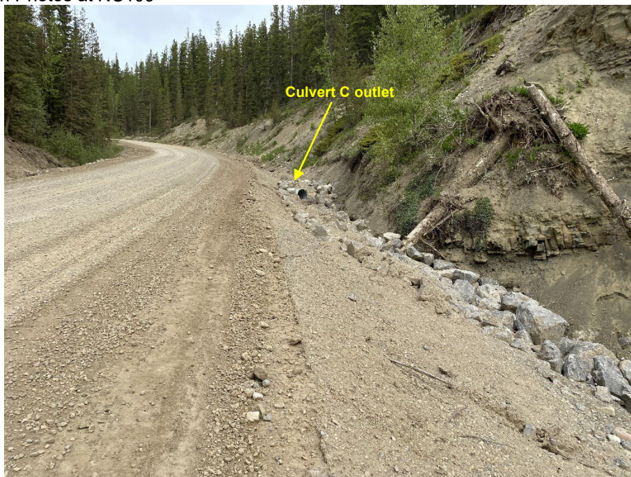
Photo 11: Culvert C outlet into eroded ditch lined with riprap. Looking northwest.
