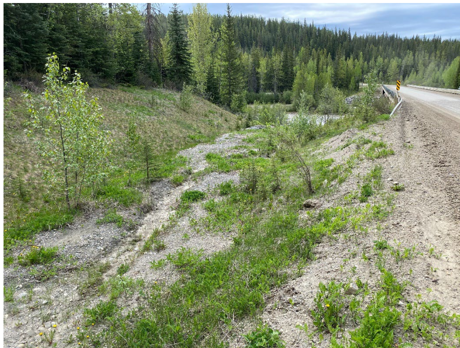
Photo 2: Erosion and sedimentation in ditch next to NBL leading up to outlet of Culvert F. Looking south.
