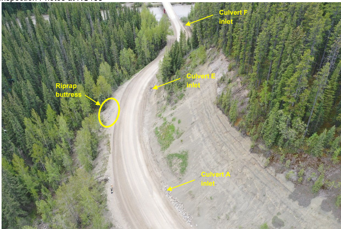
Photo 15: Overview of Highway 734 between Culvert A to the Brazeau River. Photo taken by drone, looking south.
