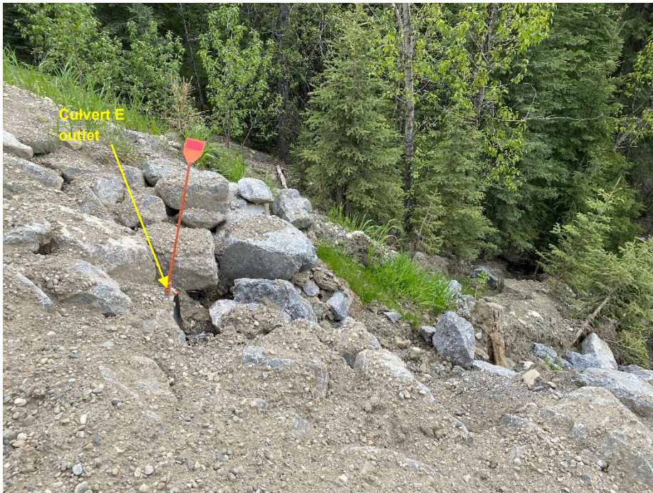
Photo 4: Bank at Culvert E lined with riprap. Erosion channel forming below. Looking northeast.
