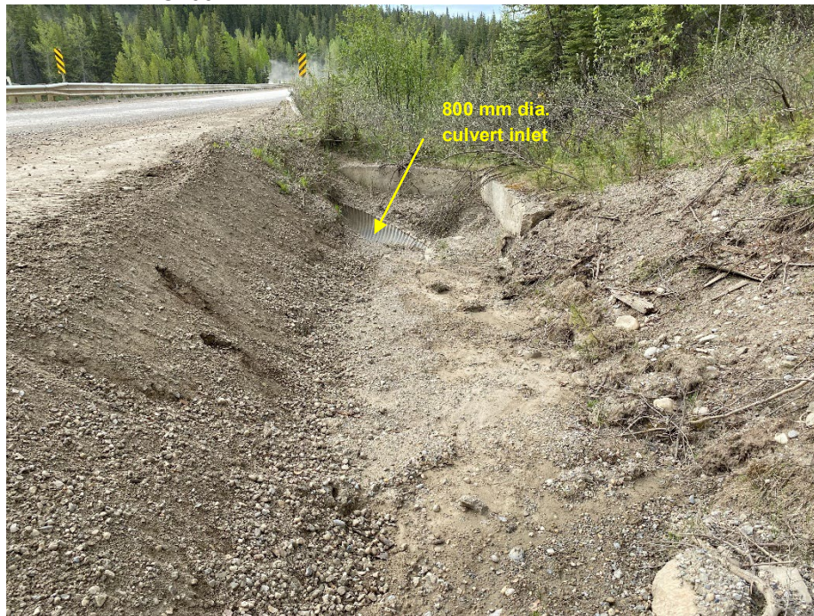
Photo 1: Erosion and sedimentation in SBL ditch leading to Culvert F. Sediment built up at beveled inlet. Looking south.
