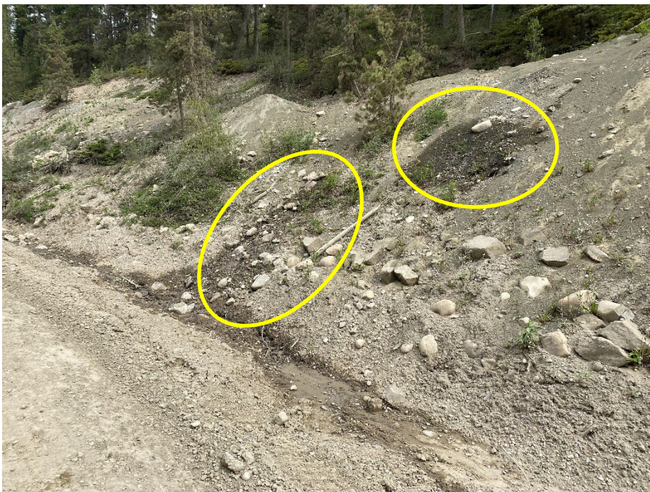
Photo 14: Seepage observed on backslope northeast of highway, south from Culvert H. Looking north.
