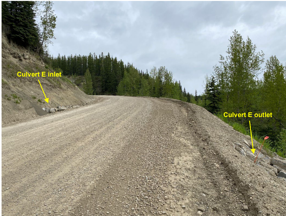
Photo 5: South end of NBL wash-out repair. Culvert E inlet and outlet lined with riprap. Looking north.
