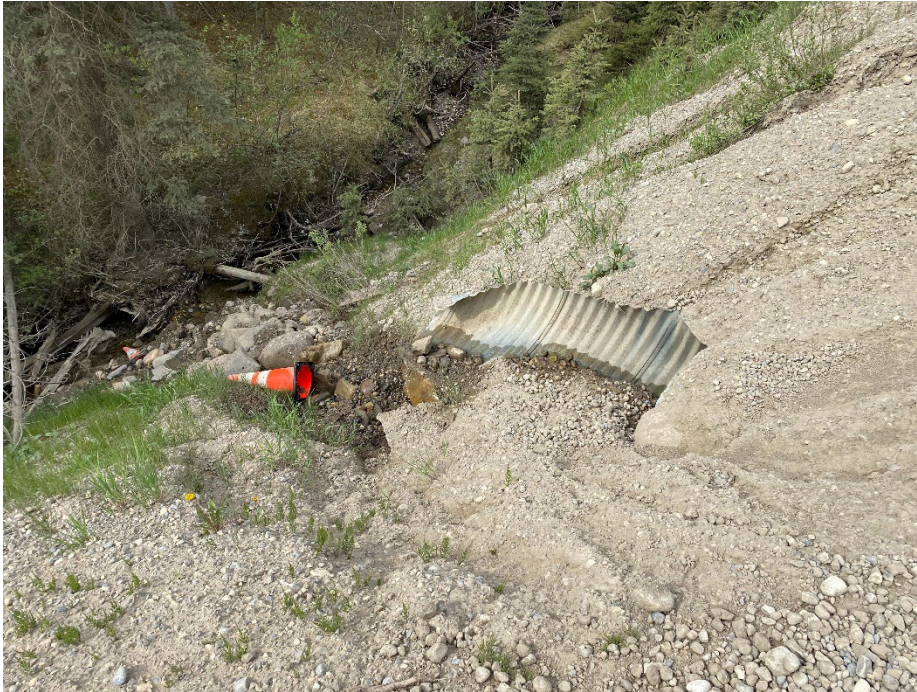
Photo 13: Outlet of Culvert H positioned above stream in south ditch. Slope above outlet washed out at the edge of the highway. Looking southwest.
