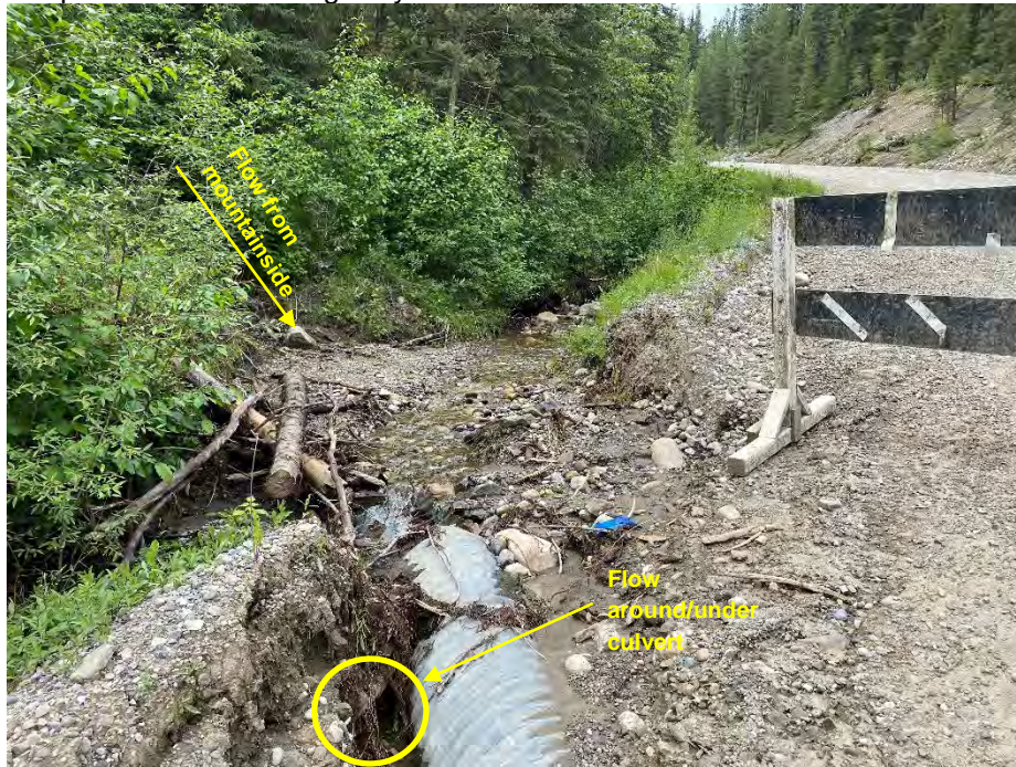
Photo 3: Culvert C inlet. Water flow from ditch and from up the mountain. Looking northwest.
