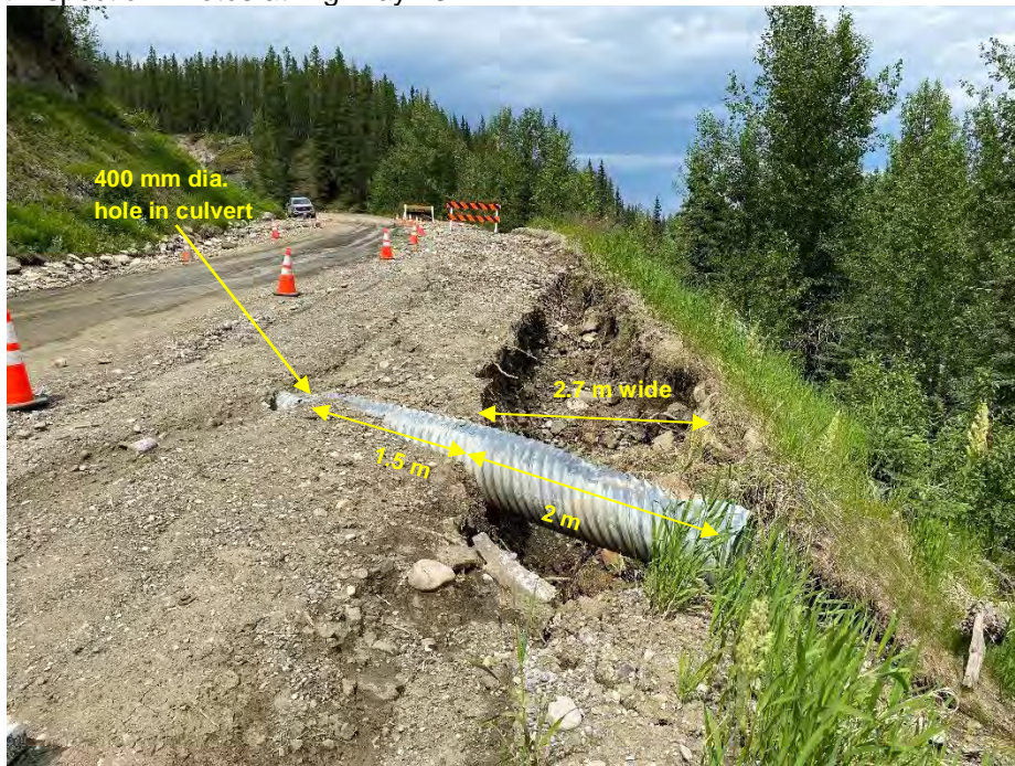
Photo 11: Erosion channel undermining Culvert E. Looking north.
