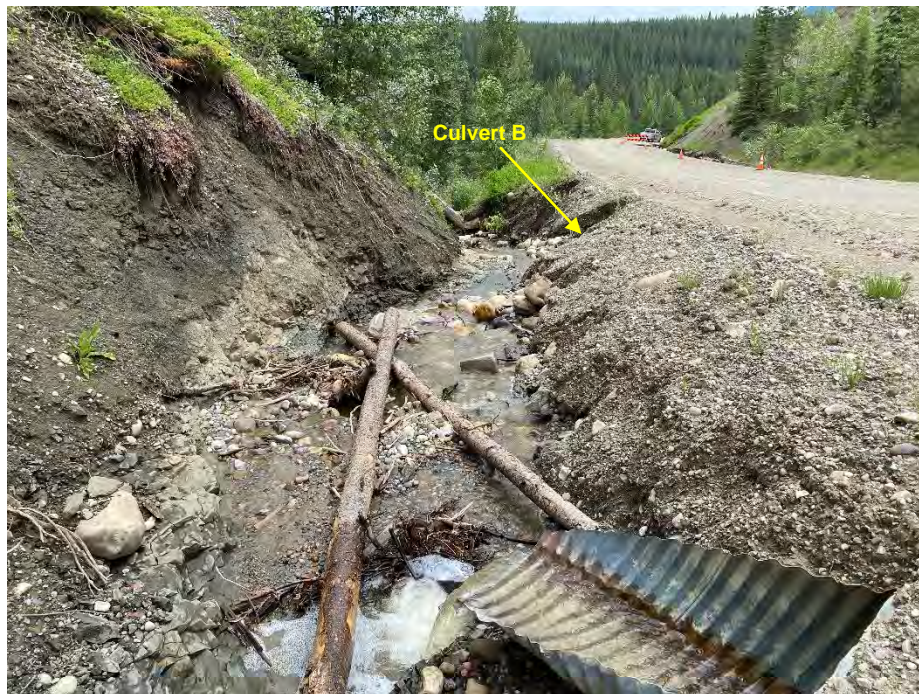
Photo 4: Culvert C discharging water to eroded NBL ditch. Looking southeast.
