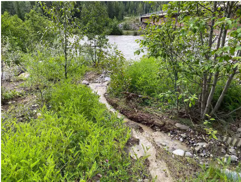
Photo 14: Culvert F discharging near Brazeau River. Note sediment buildup at beveled end. Looking south.
