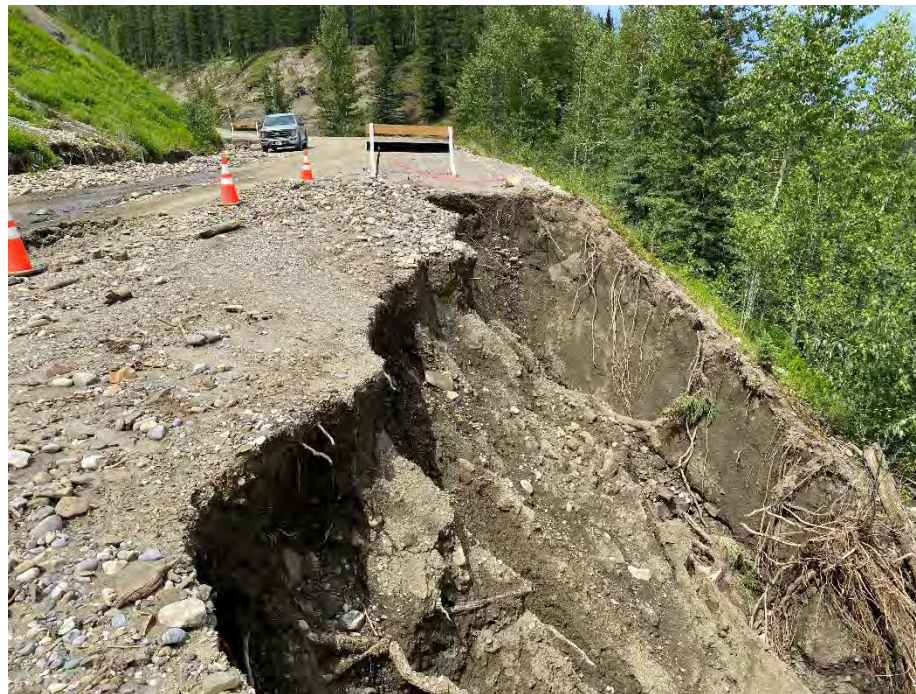
Photo 2: South end of washed-out NBL. Looking north.
