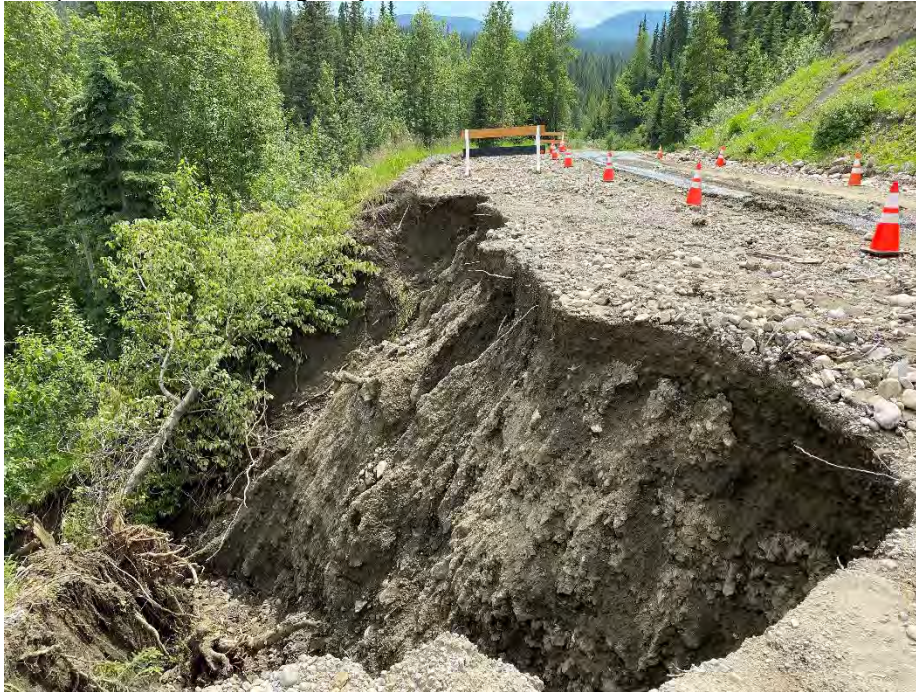
Photo 1: North end of washed-out NBL. Looking south.
