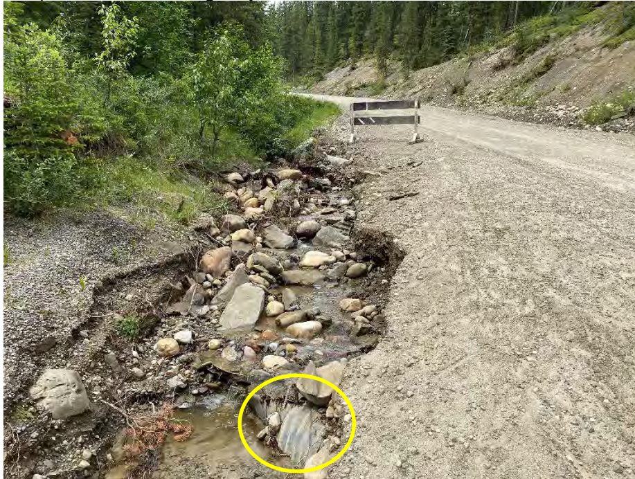
Photo 5: Culvert C buried at inlet. Severe erosion along west edge of SBL. Looking northwest.
