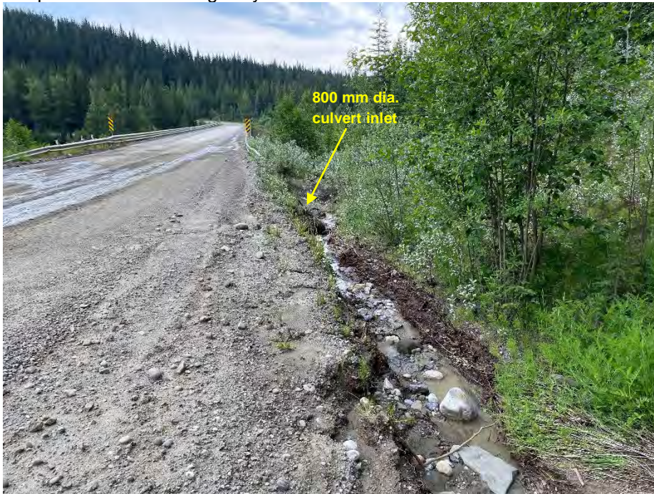
Photo 13: Erosion along SBL leading up to Culvert F. Note water flow along road coming from geohazard site uphill. Looking south.
