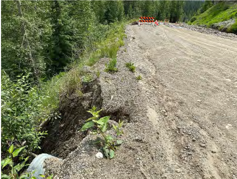
Photo 7: Overhang at Culvert A outlet. Shoulder erosion adjacent to the outlet. Looking southeast.
