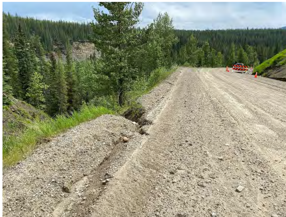
Photo 8: Eroded shoulder of NBL. Looking southeast.
