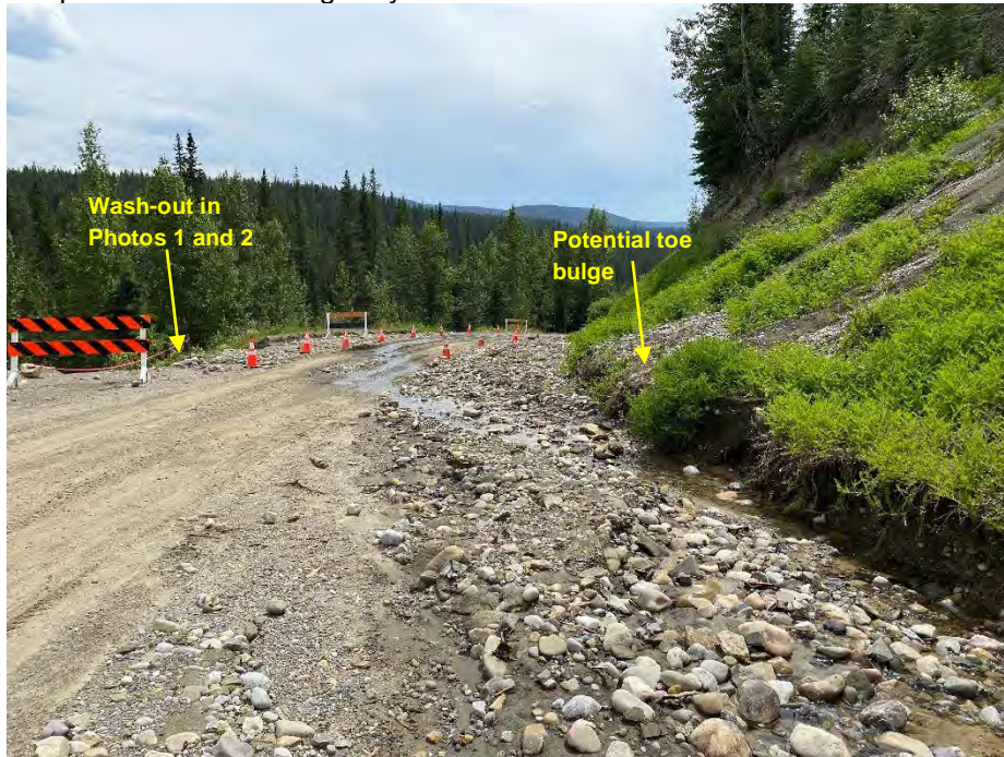
Photo 9: No ditch in SBL resulting in surface water flow towards washed-out roadway. Looking south.
