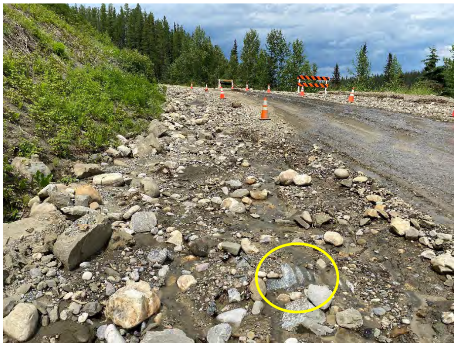
Photo 12: Culvert E inlet buried. Some water flow back to SBL ditch.
