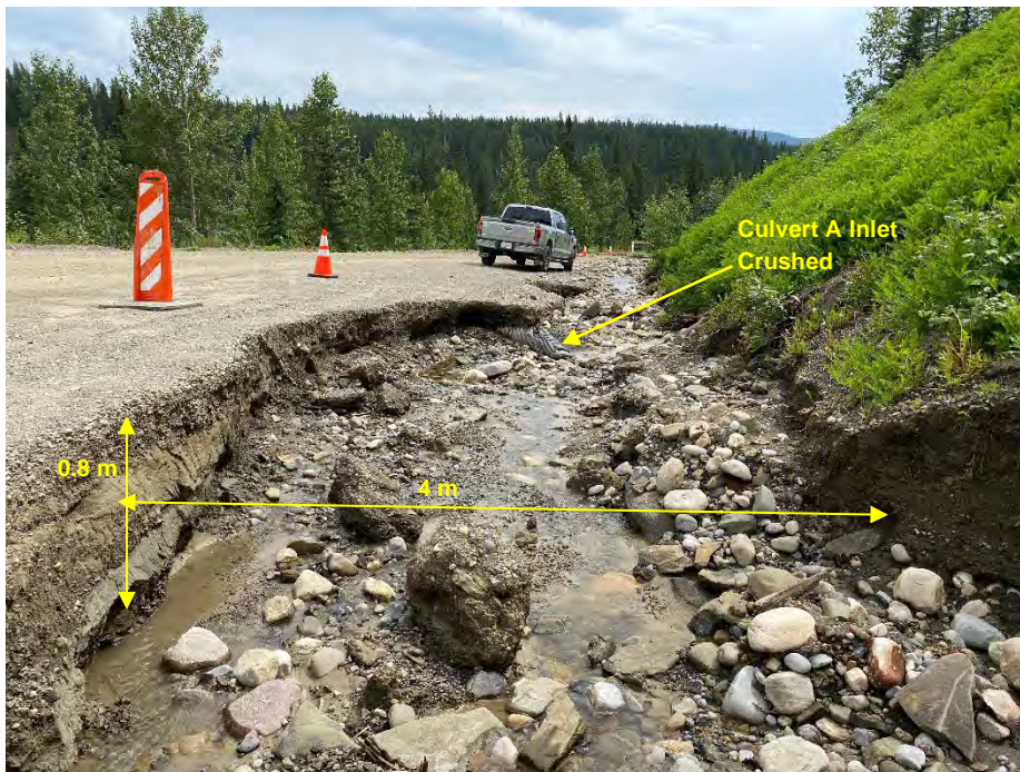
Photo 6: Severe erosion along west edge of SBL. Culvert A inlet crushed within ditch. Looking southeast.
