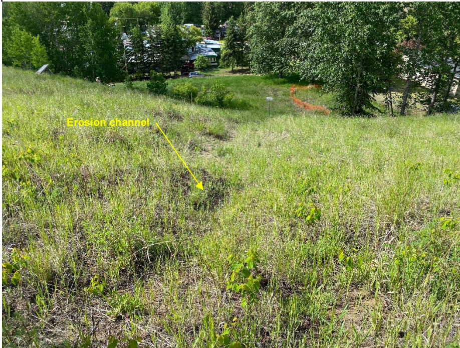
Photo 7: Erosion channel heading downslope to the bench. Looking southwest.
