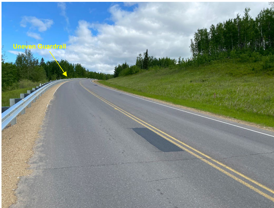
Photo 4: Pavement cracking north of mid-slope landslide. Looking northwest.
