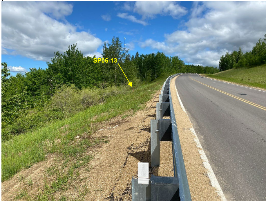
Photo 5: Landslide at uphill section. Looking northwest.
