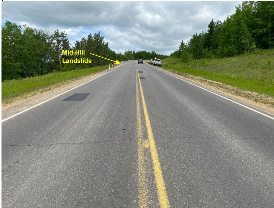
Photo 1: Pavement condition southeast of mid-hill landslide. Looking northwest.
