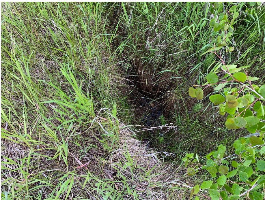
Photo 8: Sinkhole southeast from the utility box in the east ditch near the mid-hill landslide area. Looking north.
