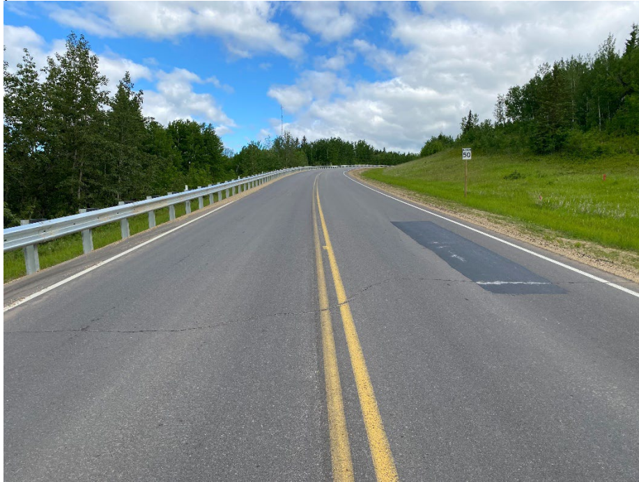
Photo 3: Cracks reflecting through pavement repair at south extent of mid-slope landslide. Looking northwest.
