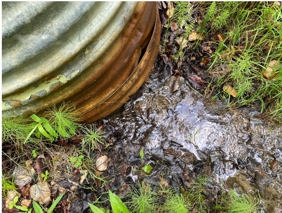
Photo 2: Pooling/flowing water adjacent to MH#1. Water entering culvert at ground surface. Looking northeast.
