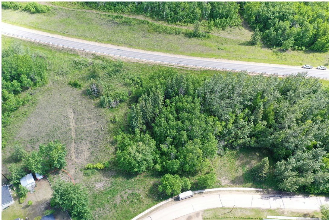
Photo 10: Overview of slide areas on highway embankment. Looking northeast.
