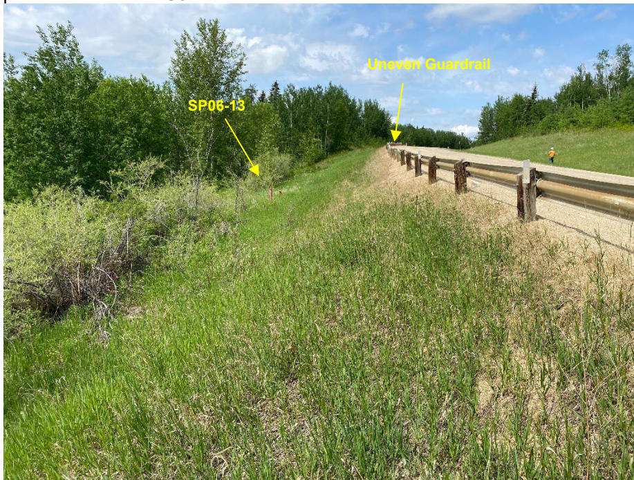
Photo 5: Landslide at uphill section. Looking northwest.
