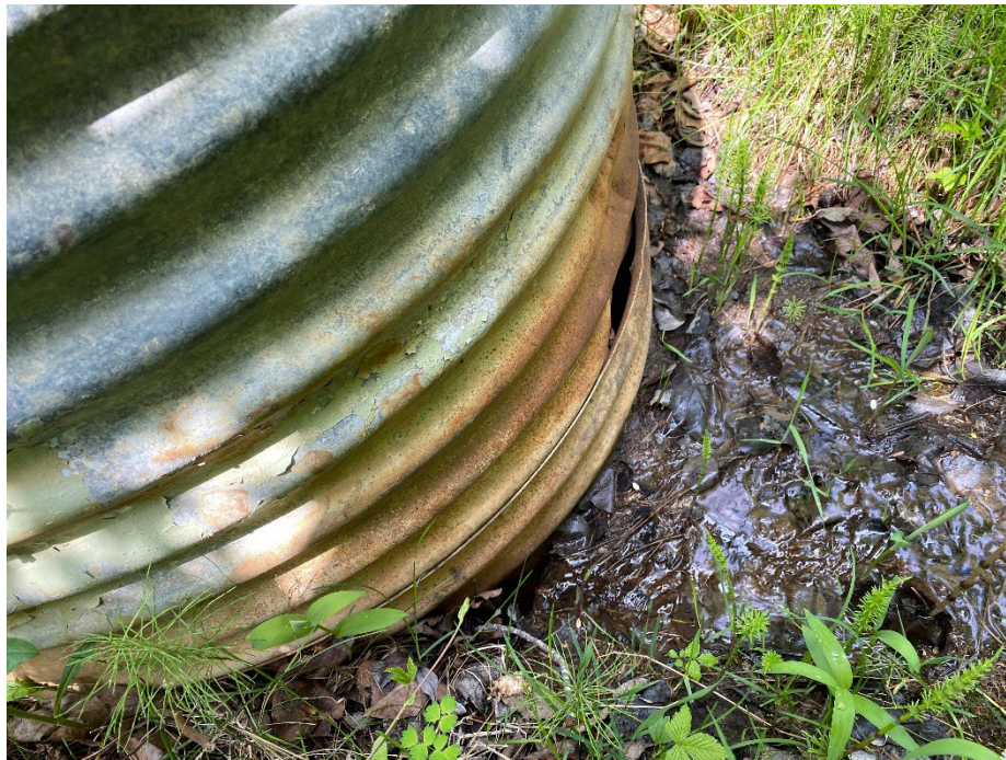
Photo 2: Pooling/flowing water adjacent to MH#1. Water entering culvert at ground surface. Looking northeast.
