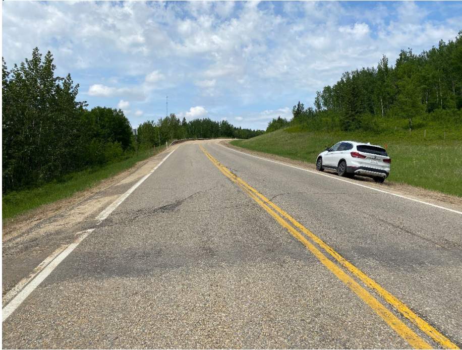
Photo 3: Pavement cracking at south extent of mid-slope landslide. Looking northwest.
