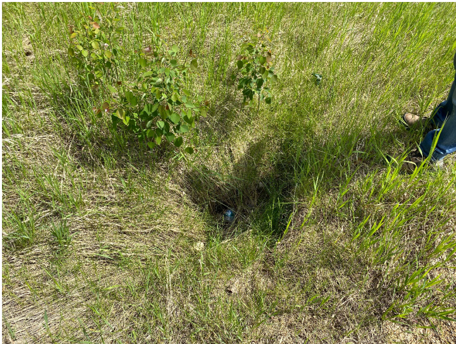
Photo 8: New sinkhole southeast from the utility box in the east ditch near the mid-hill landslide area. Looking northeast.
