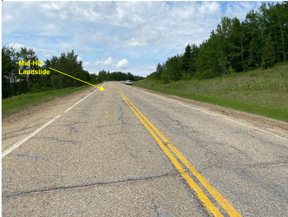
Photo 1: Pavement cracking southeast of mid-hill landslide. Looking northwest.
