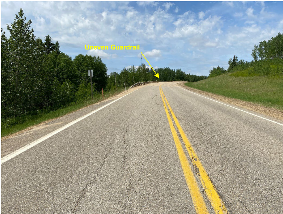
Photo 4: Pavement cracking at mid to north extent of mid-slope landslide. Looking northwest.
