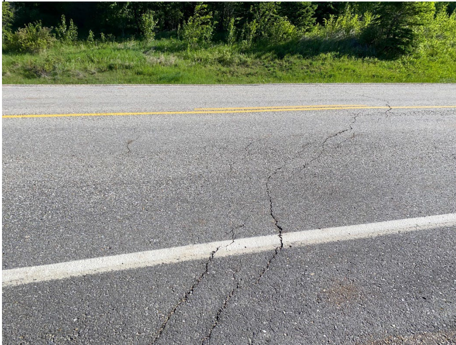
Photo 3: Angled pavement cracks across east bound lane. Looking northeast.
