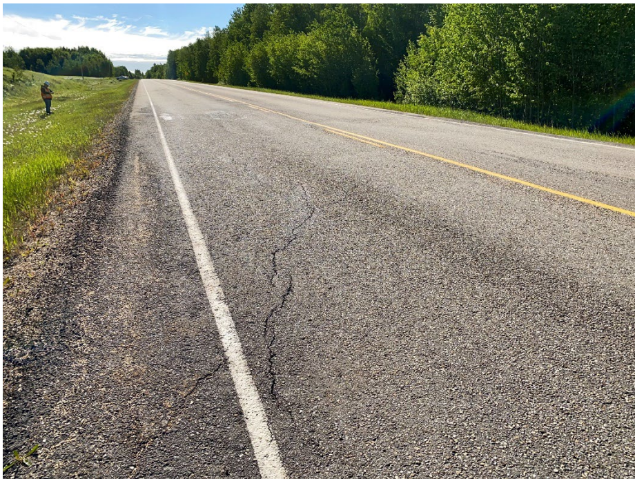
Photo 2: Pavement cracking in west bound lane. Looking east.
