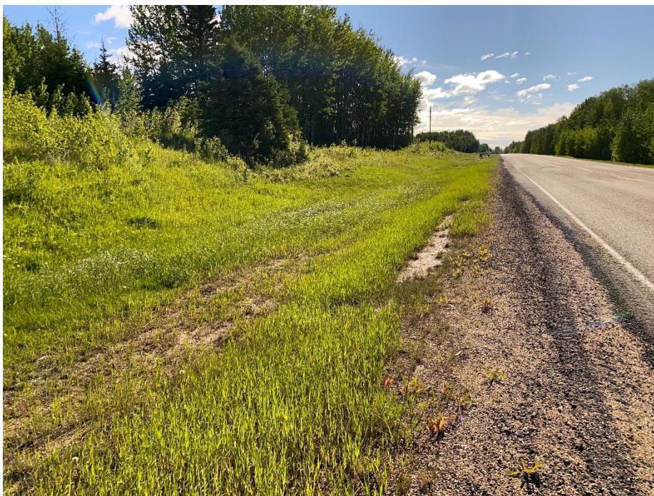
Photo 4: Minor erosion and sedimentation in north ditch. Looking east.
