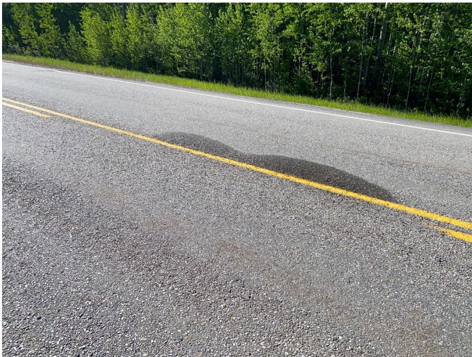
Photo 6: Possible seepage near centerline across from power pole. Looking southeast.
