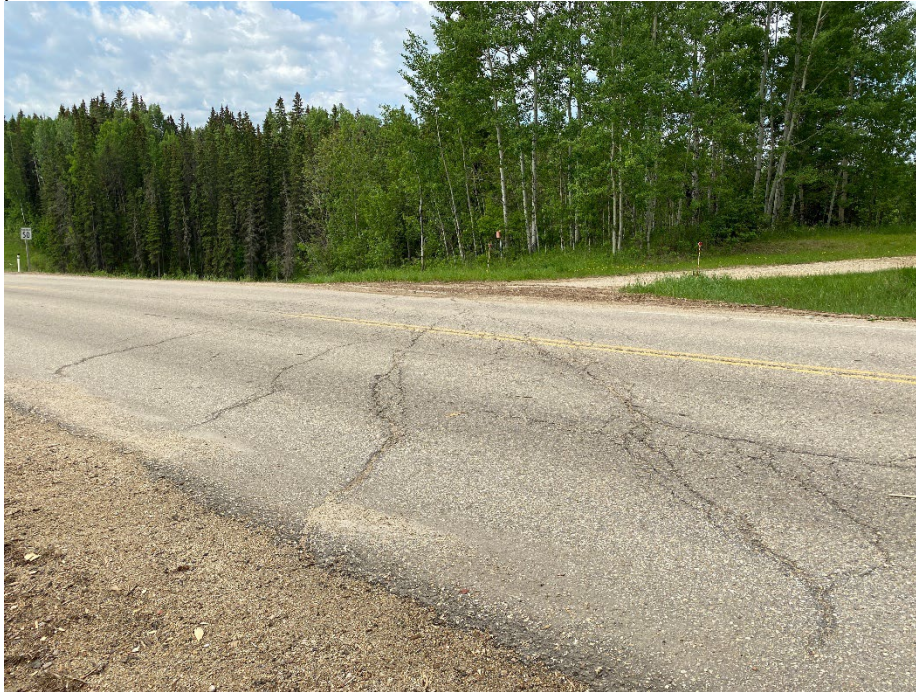
Photo 1: Pavement cracks at north portion of site at road to residence. Looking southwest.
