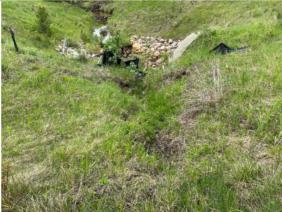
Photo 7: Erosion upslope from culvert inlet. Looking north.
