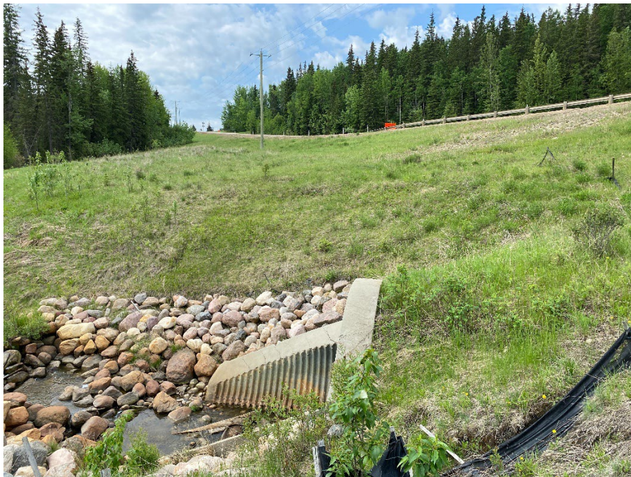
Photo 8: Skin slides south of culvert inlet. Looking southwest.
