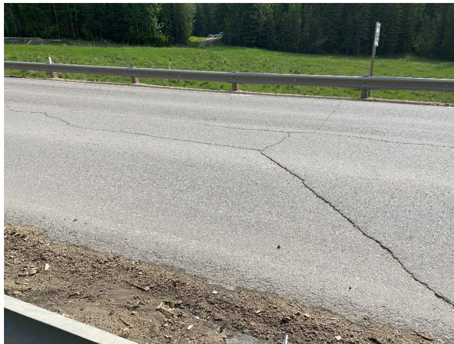
Photo 2: Pavement cracks upslope from SI19-01. Looking northeast.
