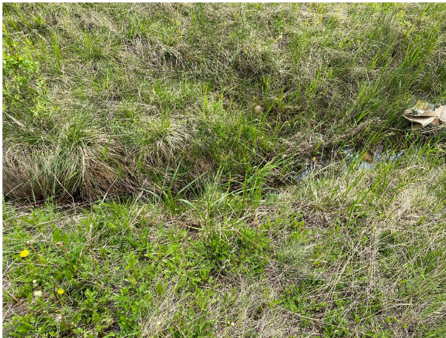
Photo 6: Erosion gully in the east ditch, north from culvert inlet. Looking east.
