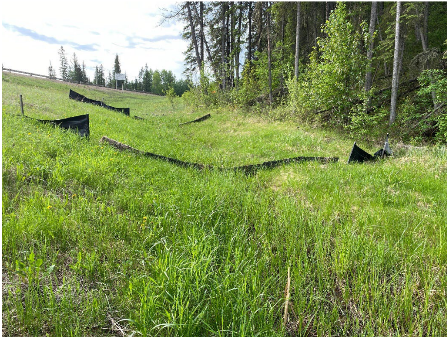
Photo 4: Gullying and ponded water present through swale leading to culvert outlet. Looking southeast.
