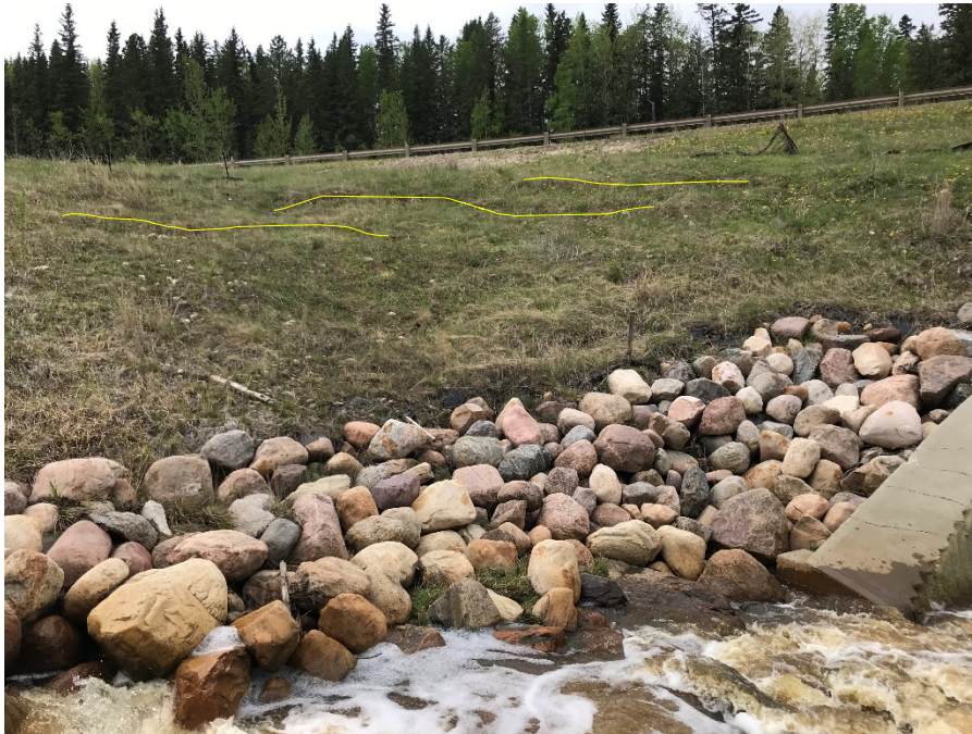
Photo 9: Tension crack developing south of culvert inlet. Looking southwest.
