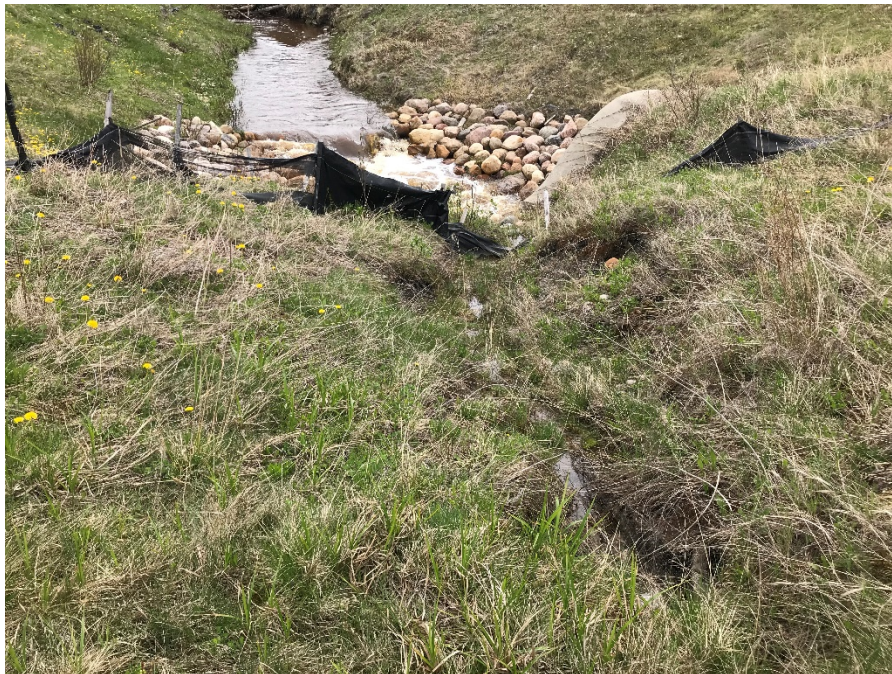
Photo 8: Erosion upslope from culvert inlet. Looking north.
