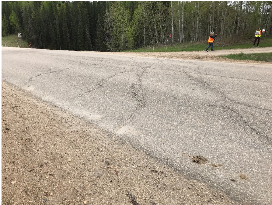
Photo 1: Pavement cracks at north portion of site at access road. Looking southwest.
