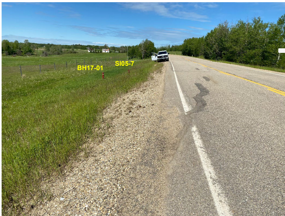
Photo 2: Pavement cracks in EB lane sealed since 2022 inspection. Looking west.
