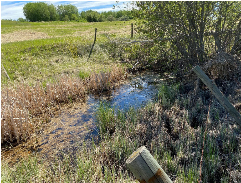
Photo 6: Ponded water at culvert inlet. Looking northeast.
