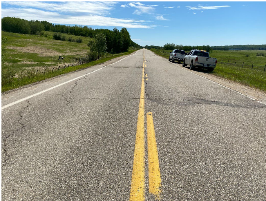
Photo 4: Pavement cracks just before west limits of 2017 patch. Looking east.
