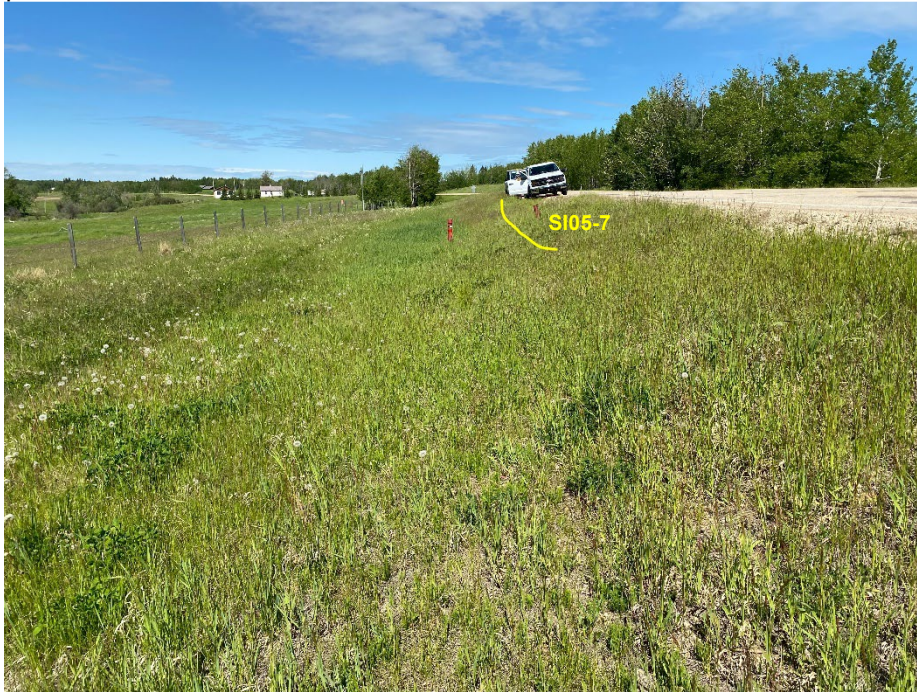
Photo 5: Potential bulging near SI05-7. Looking northwest.
