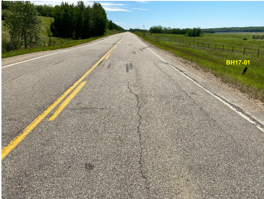
Photo 3: Cracks and skid marks on Highway 633. Looking east.
