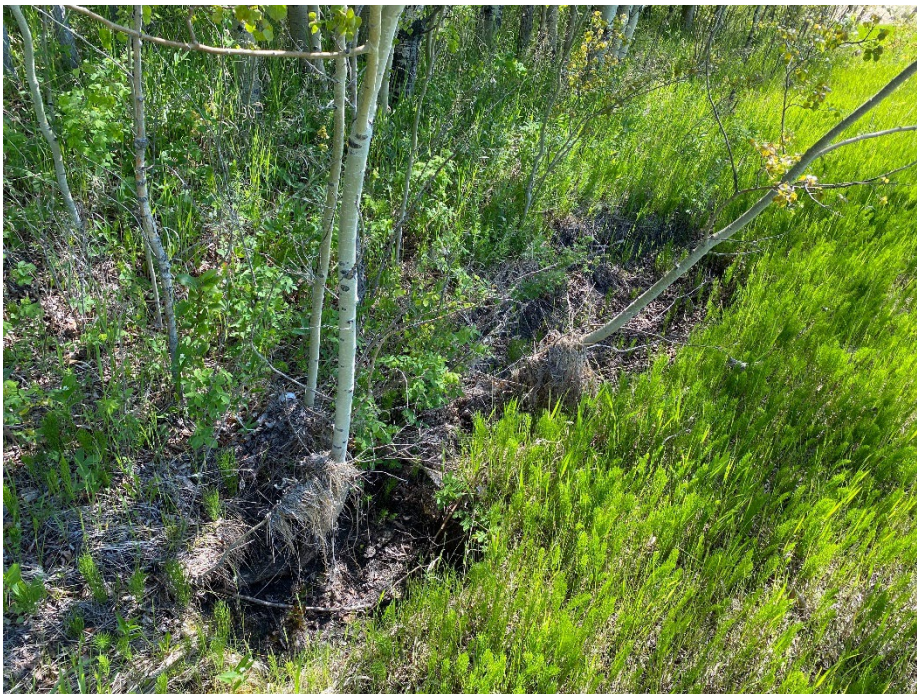
Photo 8: Erosion gully along north ditch of Highway 633. Looking east.
