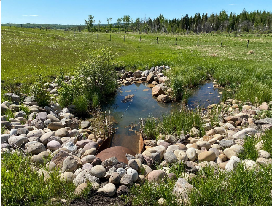
Photo 7: Ponded water at culvert outlet. Looking south.
