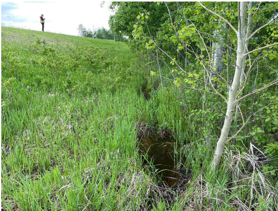
Photo 8: Erosion gully along north ditch of Highway 633. Looking southwest.
