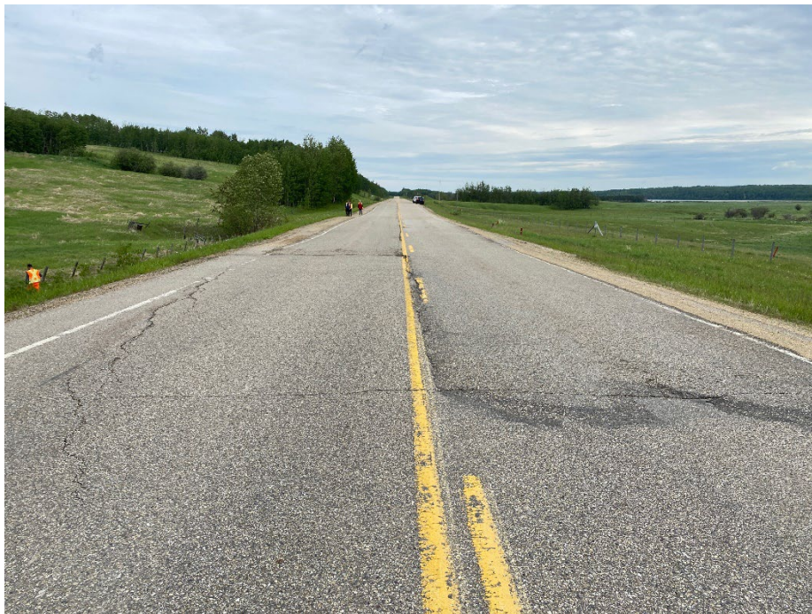
Photo 4: Pavement cracks at west limits of 2017 patch. Looking east.
