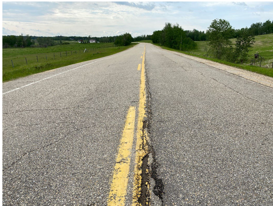
Photo 2: Pavement cracks along Highway 633. Looking west.
