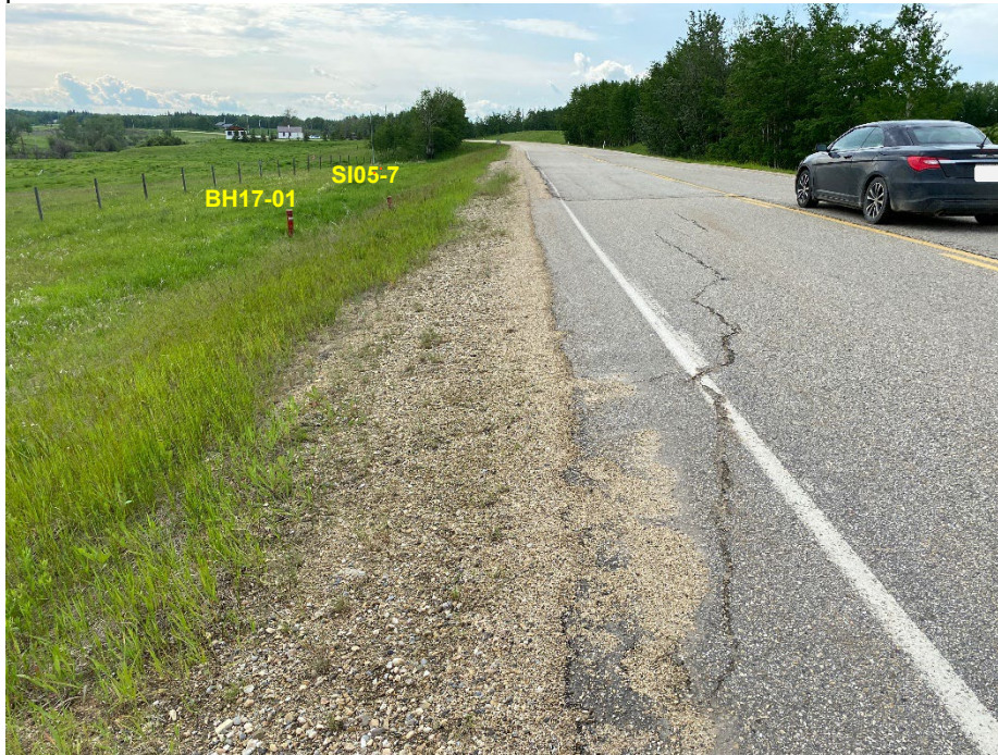
Photo 3: Pavement cracks along Highway 633. Looking west.
