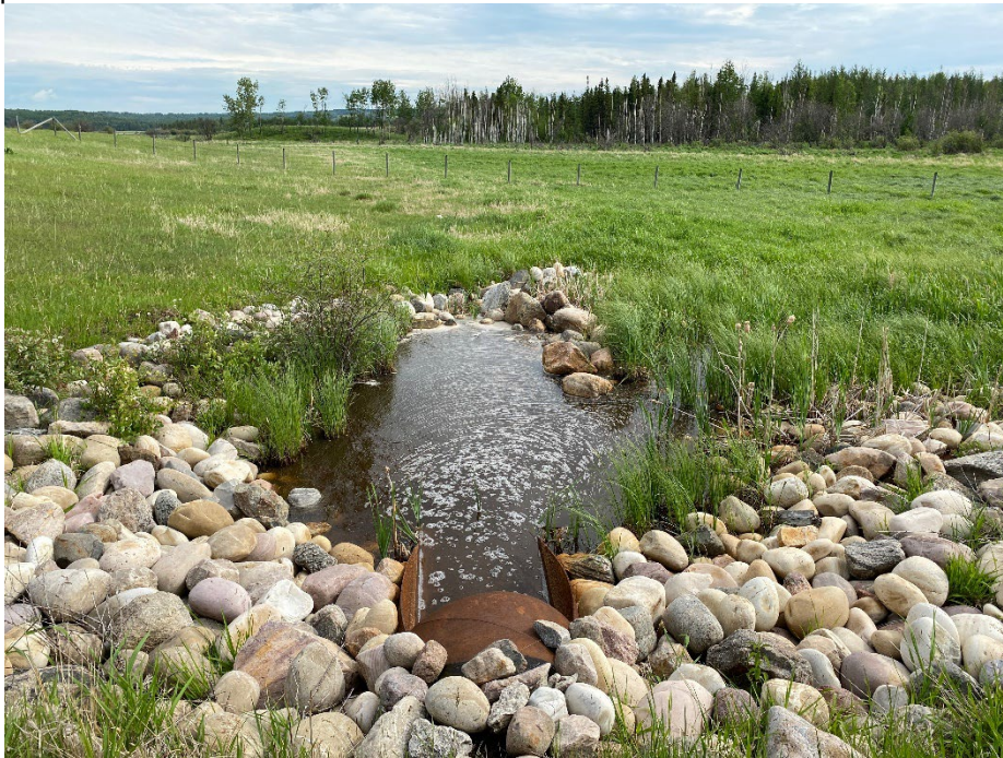
Photo 7: Ponded water at culvert inlet in the south. Looking south.
