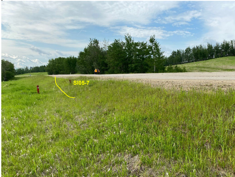
Photo 5: Potential bulging near SI05-7. Looking northwest.
