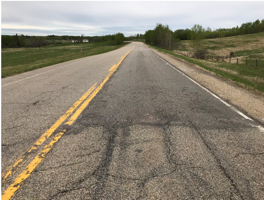
Photo 1: Pavement cracks at east limits of 2017 patch. Looking west.
