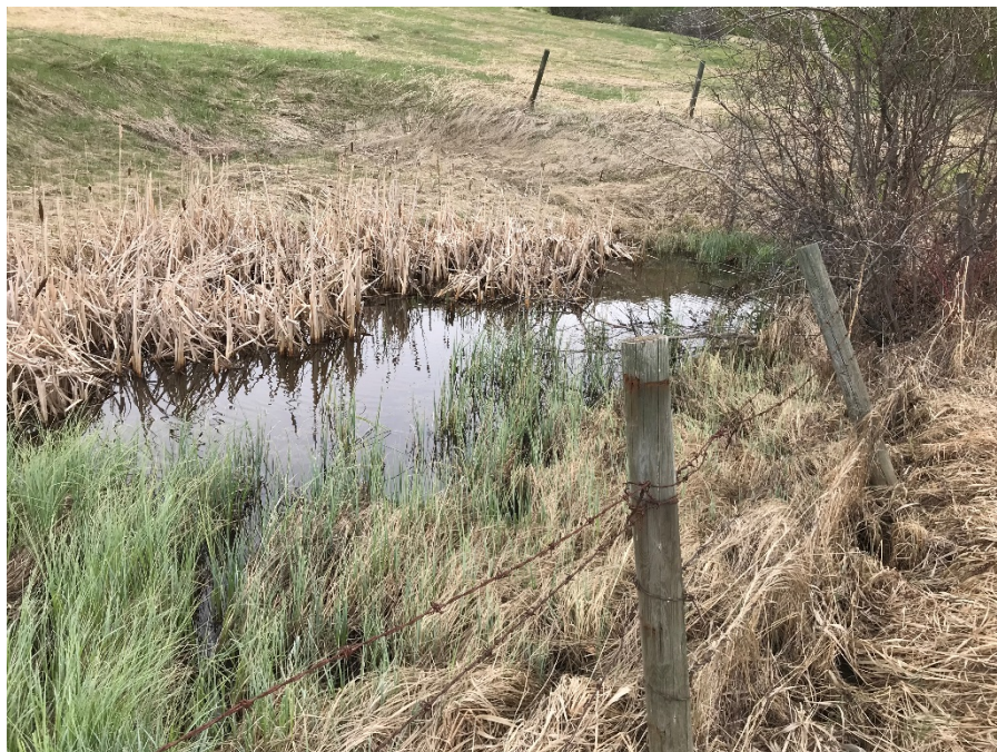
Photo 6: Ponded water at culvert inlet in the north. Looking northeast.
