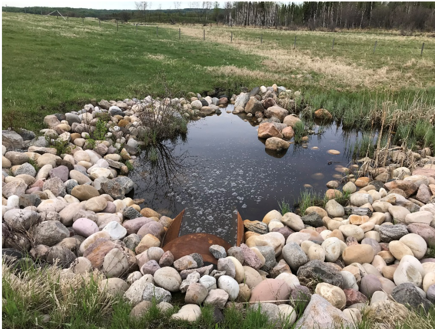
Photo 7: Ponded water at culvert outlet in the south. Looking south.
