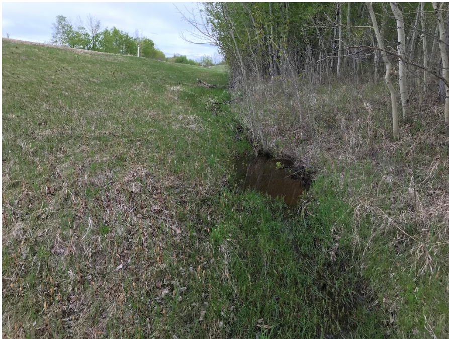
Photo 8: Erosion gully along north ditch of Highway 633. Looking west.
