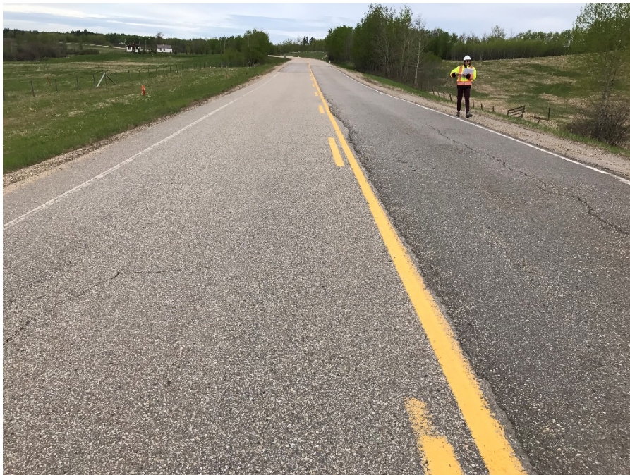
Photo 2: Pavement cracks along Highway 633. Looking west.
