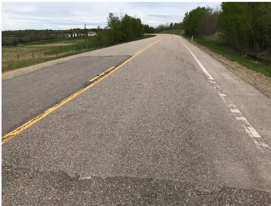
Photo 4: Pavement cracks at west limits of 2017 patch. Looking west.
