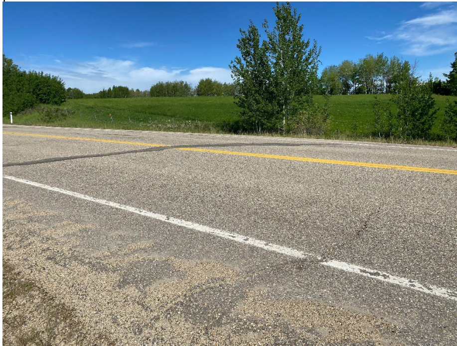
Photo 1: Sealed circular crack approximately 40 m west of SI05-1 and smaller circular crack in EBL. Looking northwest.
