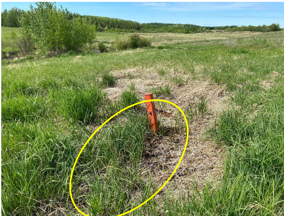
Photo 6: Settlement around BH17-02 on the south embankment. Looking west.
