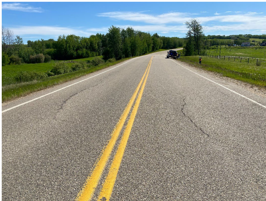
Photo 2: Semi-circular pavement cracks about 10 m east of Photo 1. Looking northeast.
