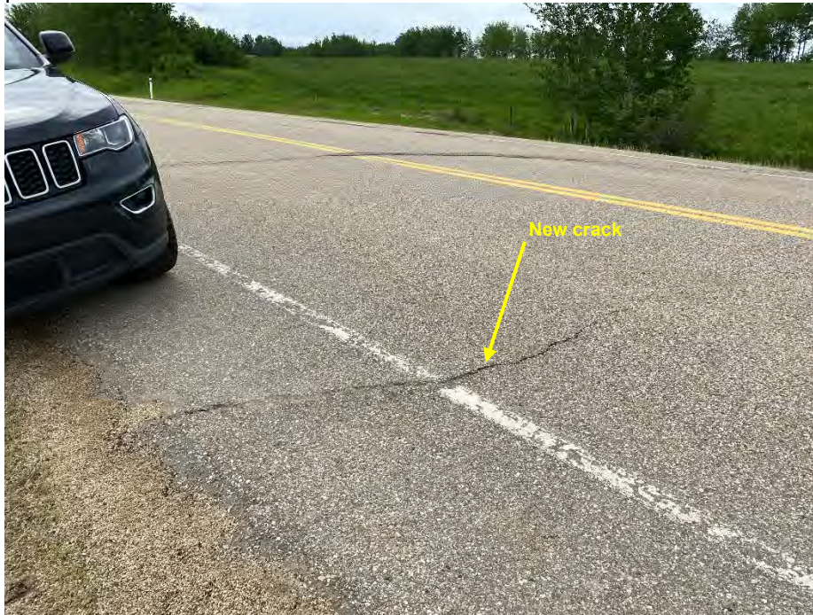
Photo 1: Circular crack approximately 40 m west of SI05-1 and new crack forming in EBL. Looking northwest.
