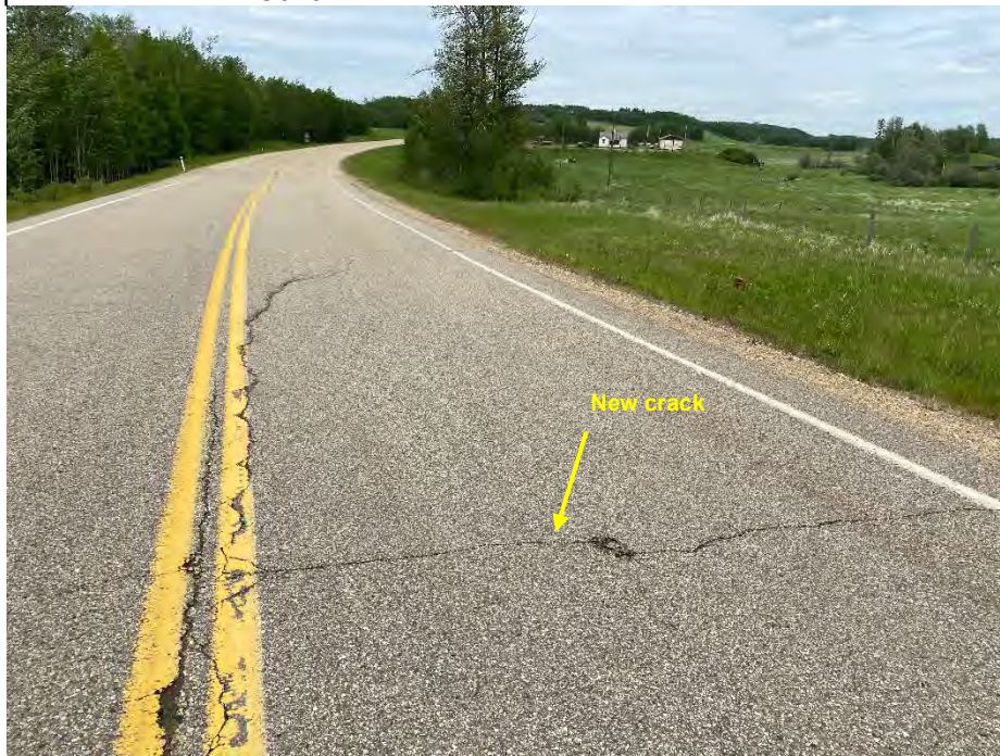
Photo 5: Semi-circular crack along C/L and EBL lane north of BH17-01. New transverse cracking. Looking east.
