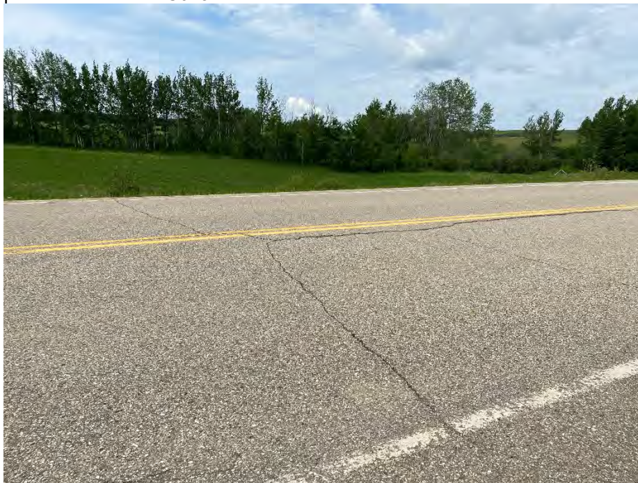
Photo 3: Pavement cracking approximately 15 m east from SI05-1. Looking north.
