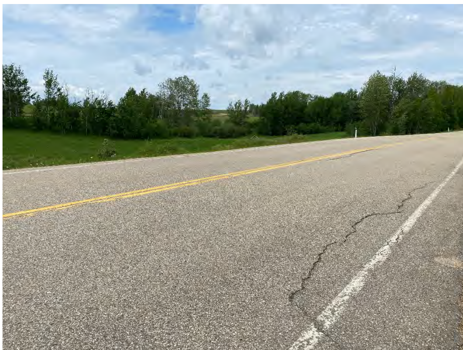
Photo 4: Crack on shoulder north of SI05-1. Looking northeast.
