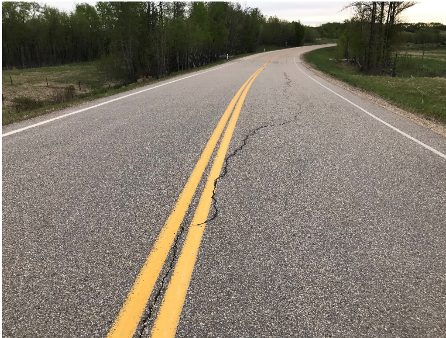
Photo 5: Semi-circular crack along C/L and eastbound lane north of BH17-01 Looking west.
