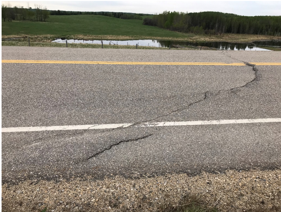
Photo 1: Circular crack approximately 40 m west of SI05-1. Looking south
