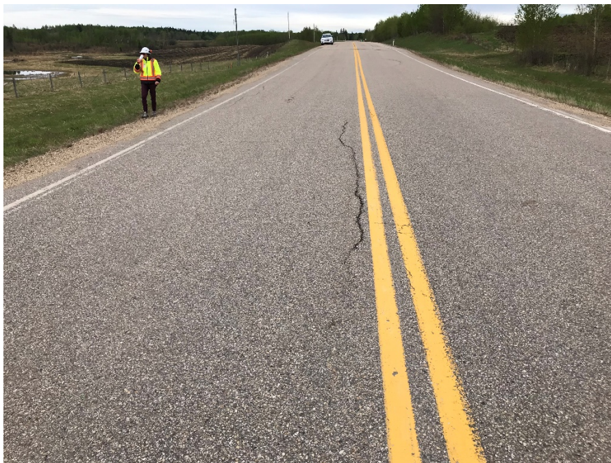
Photo 4: Cracking on eastbound lane northwest of BH17-01 Looking west.
