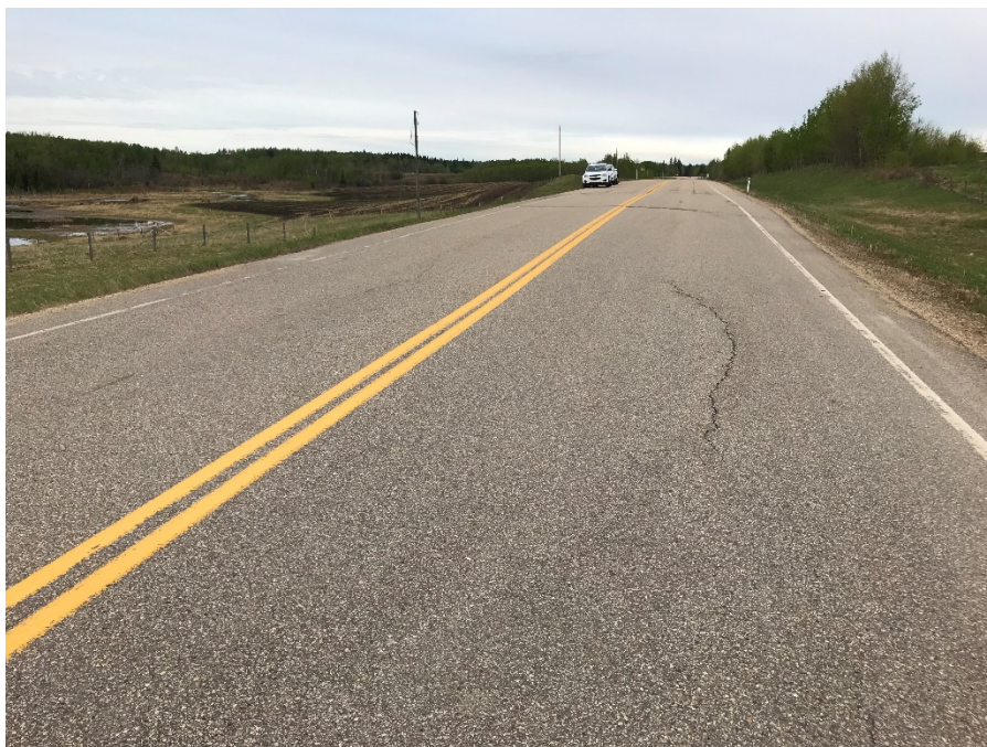
Photo 2: Semi-circular pavement crack about 10 m east of Photo 1. Looking west.
