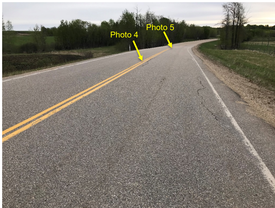
Photo 3: Crack on shoulder north of S105-1 unchanged. Looking east.
