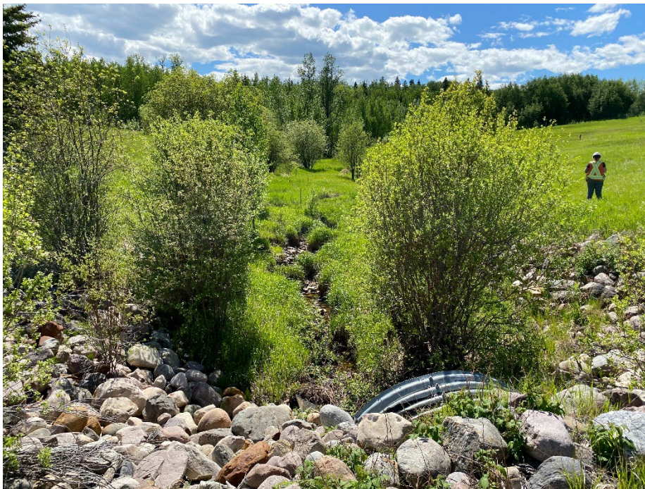
Photo 8: Looking down channel beyond culvert outlet on south side of highway. Facing southwest.
