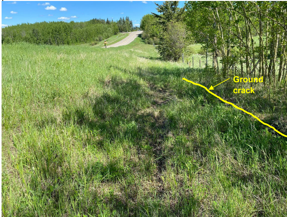
Photo 5: South ditch, looking east. Ground crack visible near fence line, possibly due to removal of silt fence.
