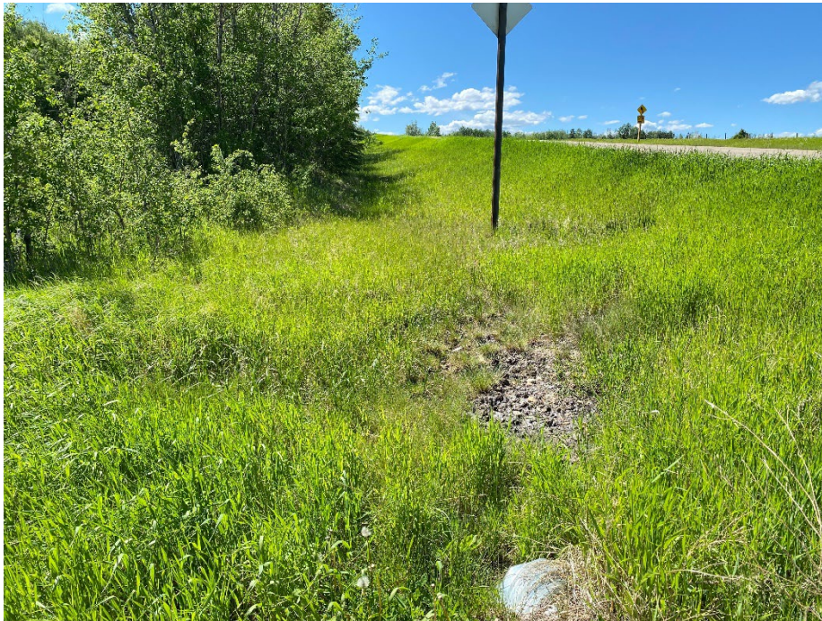
Photo 4: Erosion at west end of culvert across property access road. Looking west.
